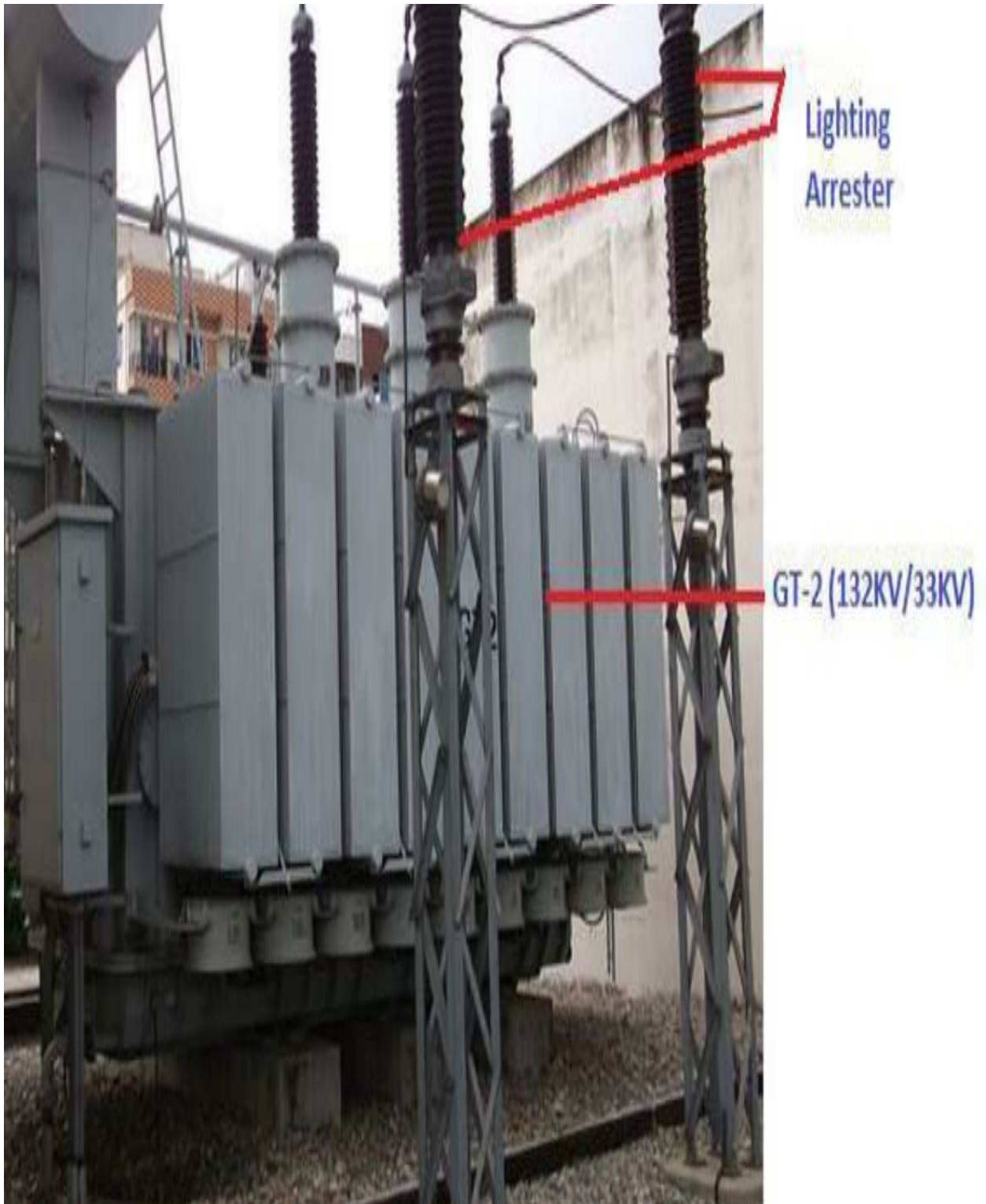
Figure 5.8: Lighting Arrester of GT-2 at Mirpur grid-substation.
