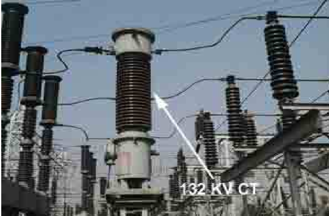
Figure 5.6: Current transformer at Mirpur grid-substation.
