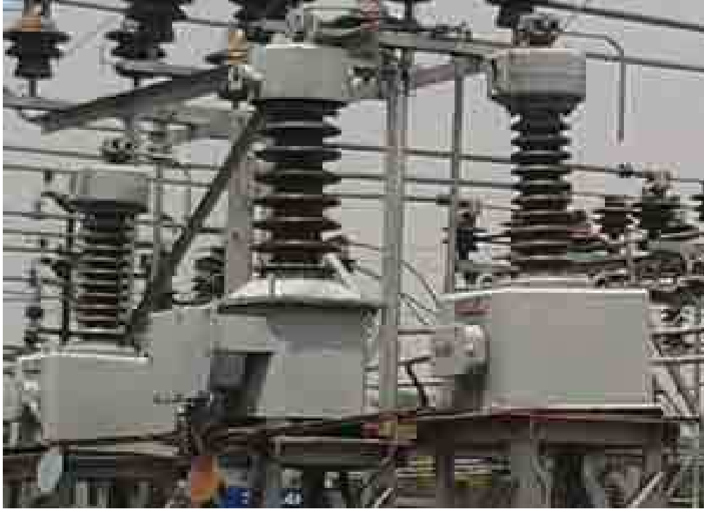
Figure 5.7: Potential transformer at Mirpur grid-substation.
