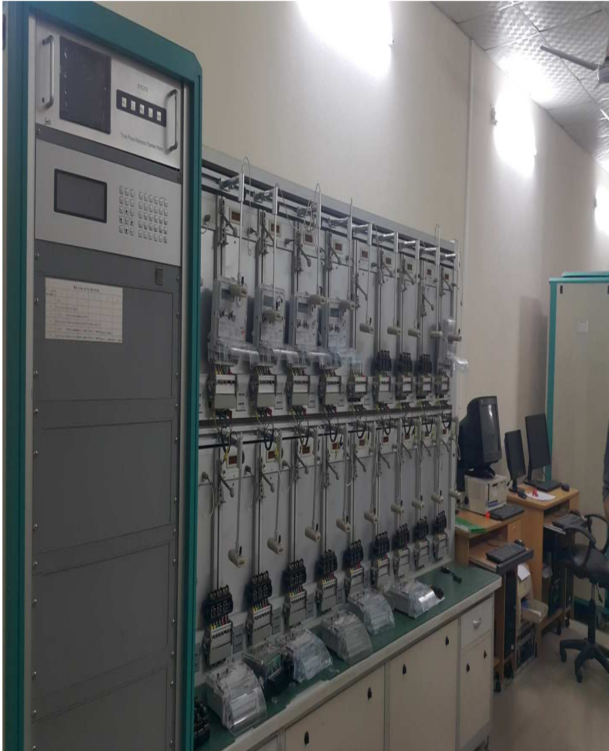
Figure 7.4: Meter testing board.
