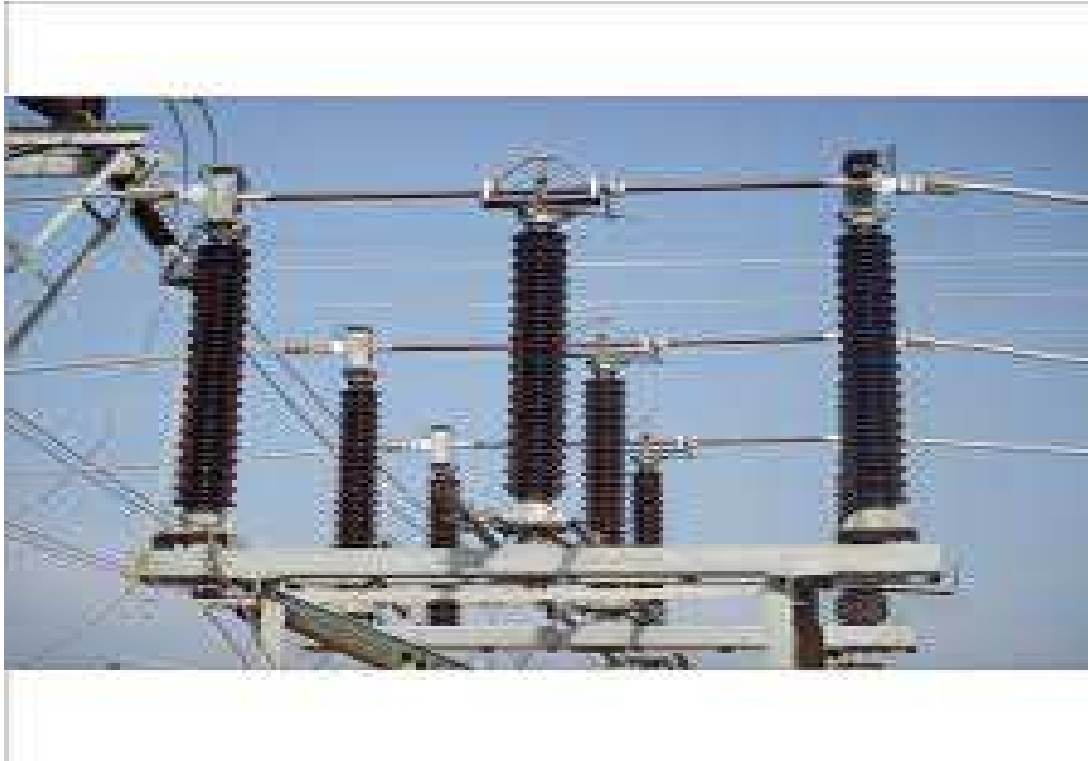
Figure 5.5: Line isolator at Mirpur grid-substation.
