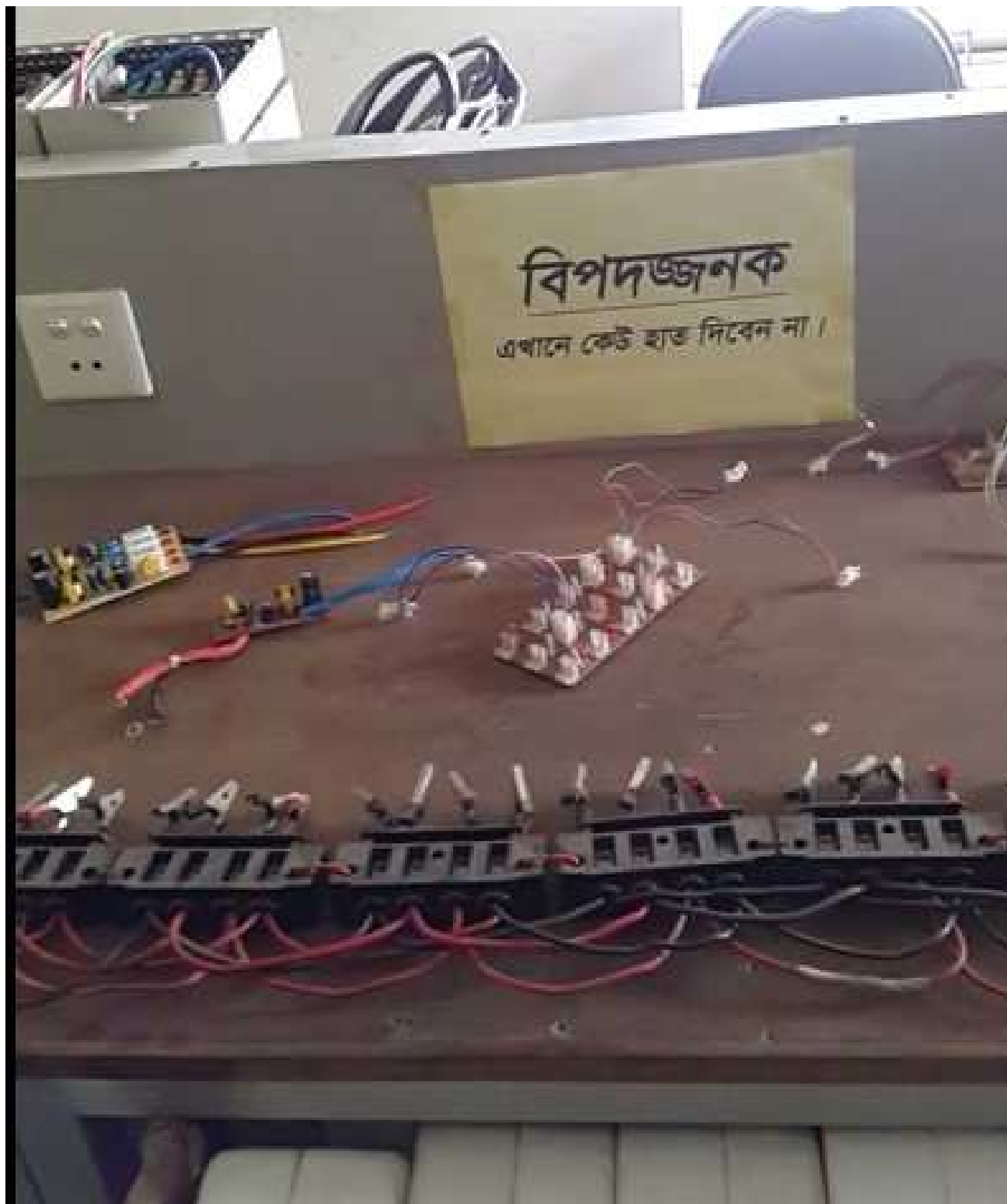
Figure 7.3: Meter testing & repairing unit.
