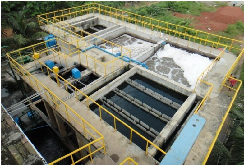
Figure 41: Effluent treatment plant in ADML
