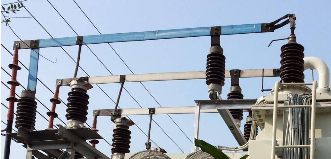
Fig 4.2: 33kV incoming source from Dagon and Damel CT, L.A, PT, HT Bushing
