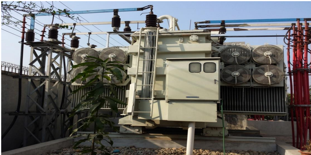
Fig 4.1: Power Transformer at Paralall pallabi Substation
