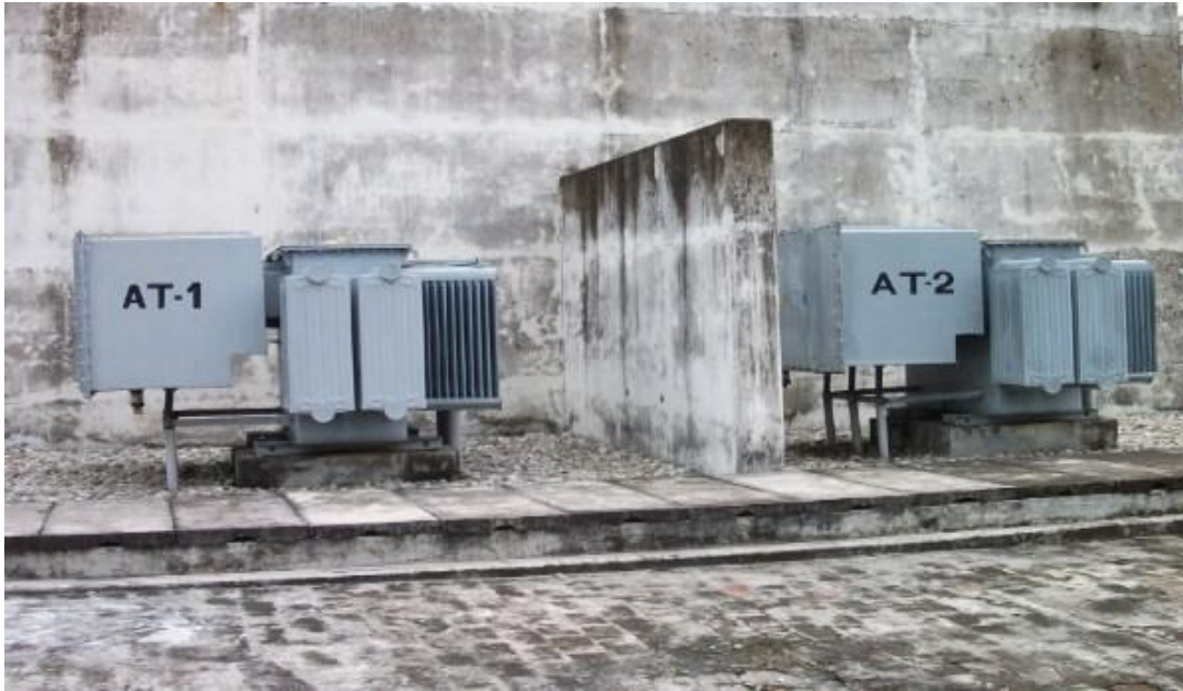
Fig 4.12: Auxiliary transformer at Pallabi-substation.
