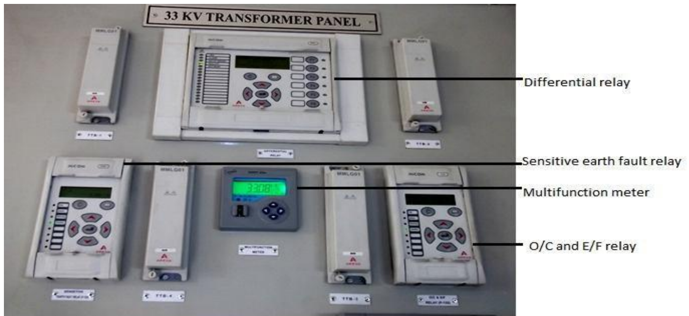
Fig 5.6: The digital relay protection on 33KV transformer panel.
