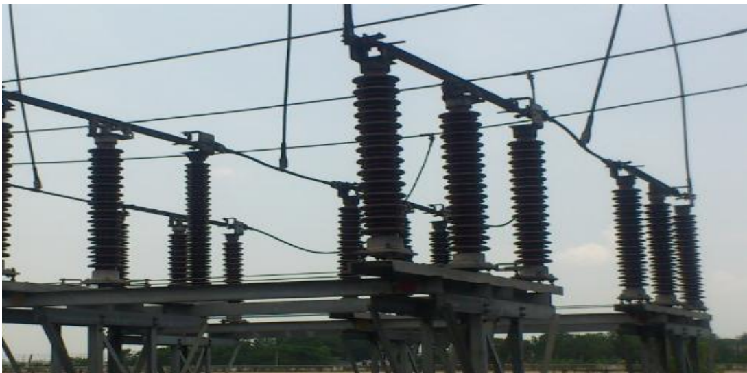
Figure 4.5.: Isolators in Pallabi Substation
