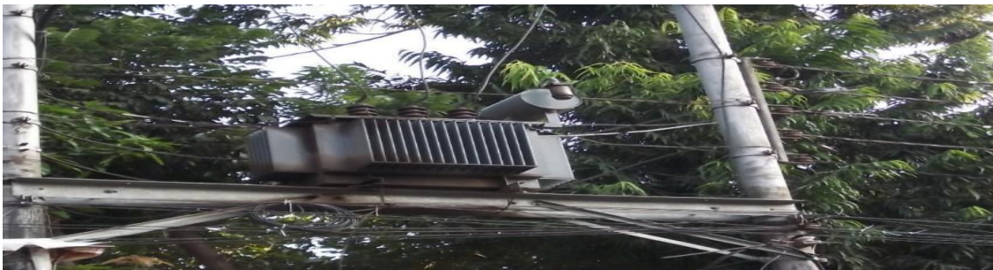
Figure 5.2: The 11/440KV distribution transformer.
