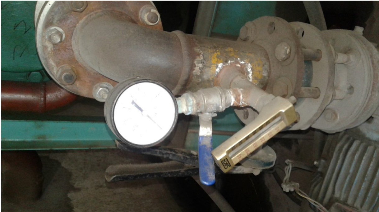
Figure 2.2.11: Pressure Gas with Metering System
