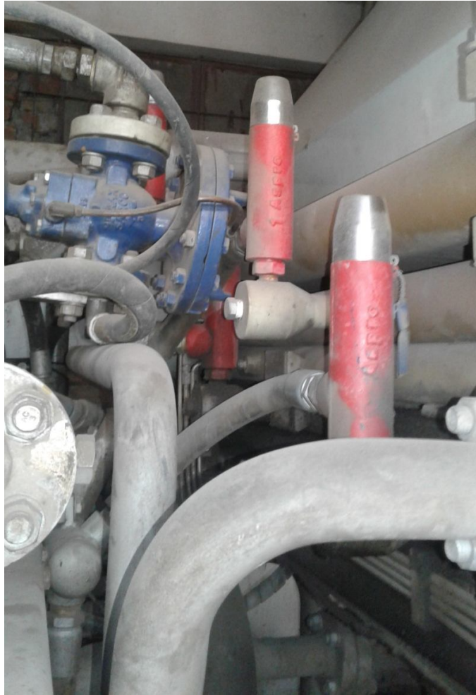
Figure 2.2.9: Safety valve with compressore machine
