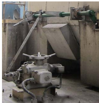
Figure 3.9.3: FD fan air flow control valve.
