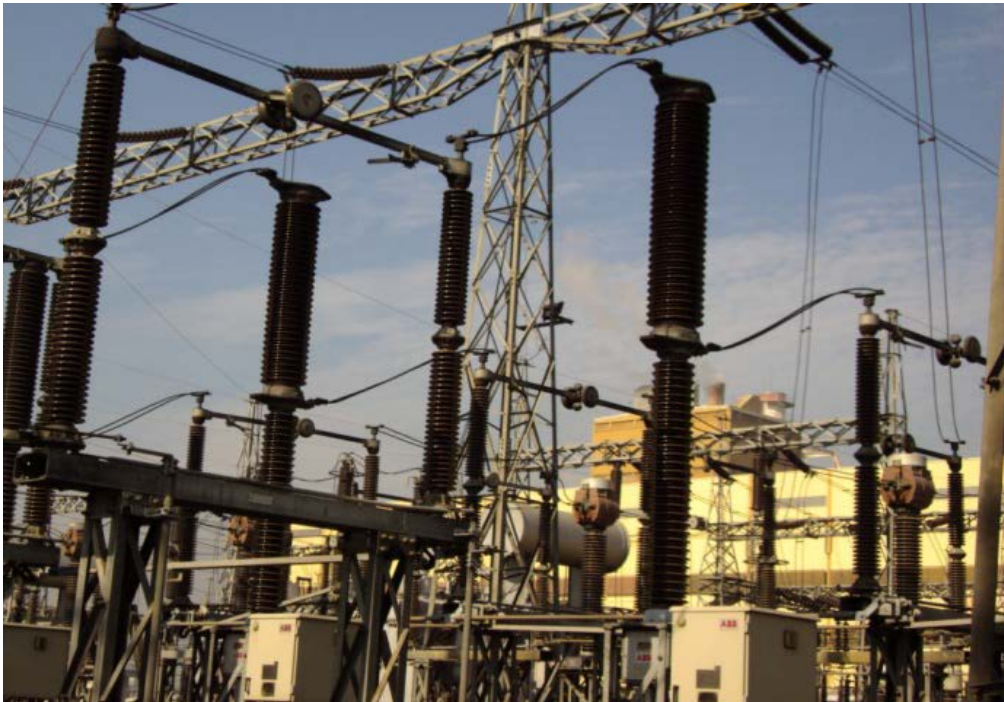
Figure 5.4.2: Oil Circuit Breaker used at APSCL Substation
