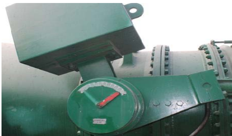
Figure 3.8.8: pressure relief valve
