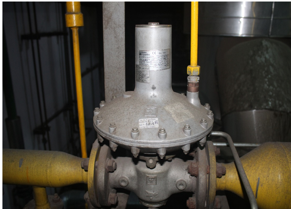
Figure 3.8.1.1: Gas pressure reducing valve.
