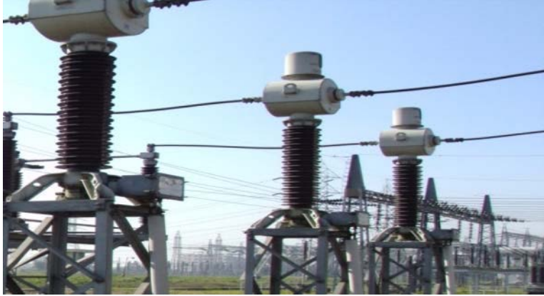
Figure 5.3.2.2: Potential Transformer used at APSCL Substation (132 kV single phase outdoor types)
