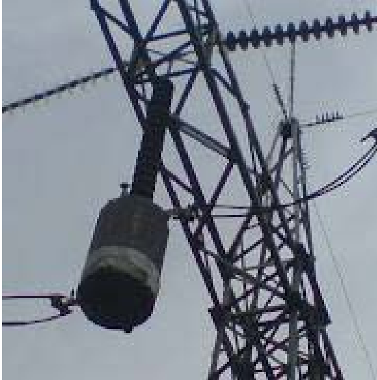
Figure 5.9: Wave trap used on APSCL substation.
