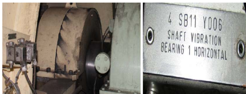
Figure 4.6.9: Shaft vibration sensor for unit 5 steam turbine connects with shaft.
