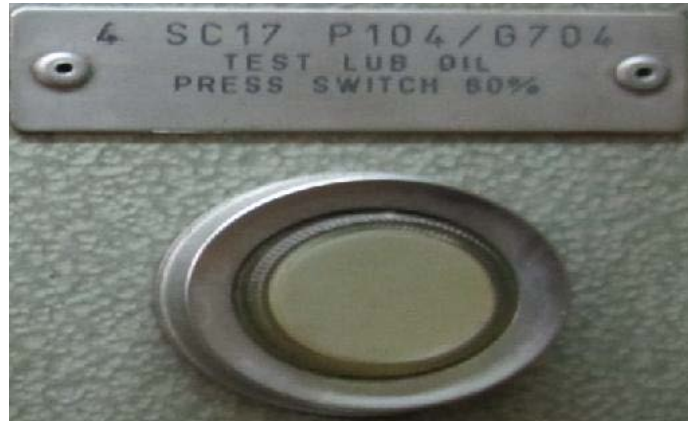
Figure 4.6.10 Shows the Lube Oil Pressure Protection Switch
