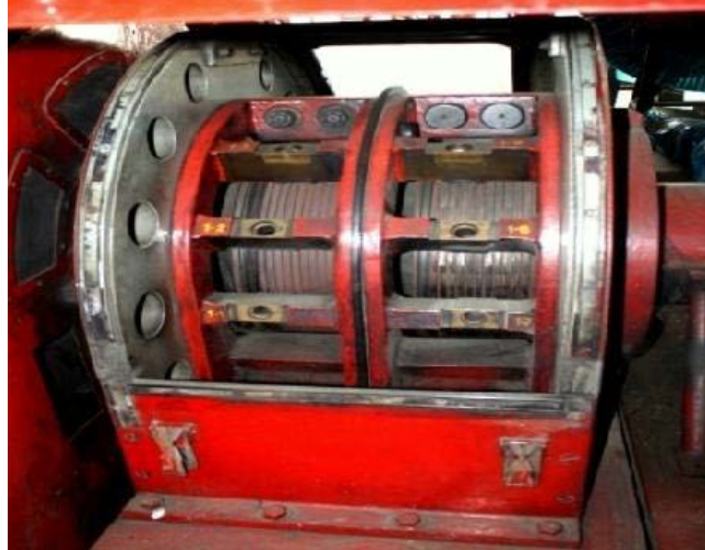
Figure 4.5.1: Pilot Generator in 150 MW generator of unit 3.
