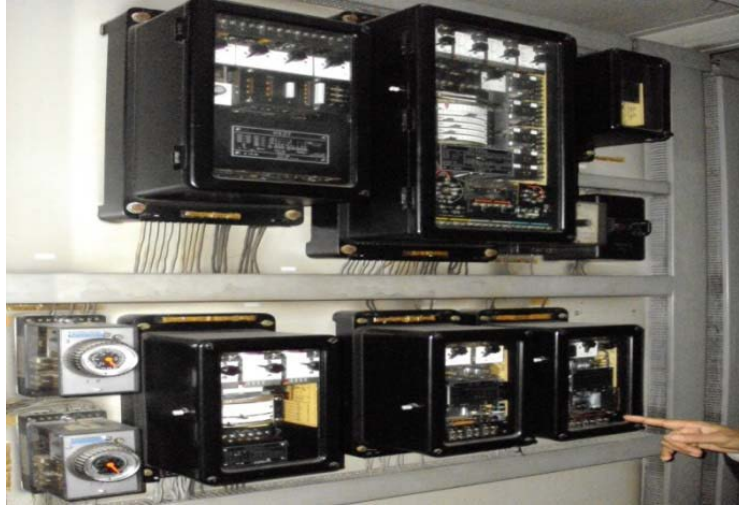
Figure5.5.1: protective relay used at APSCL
