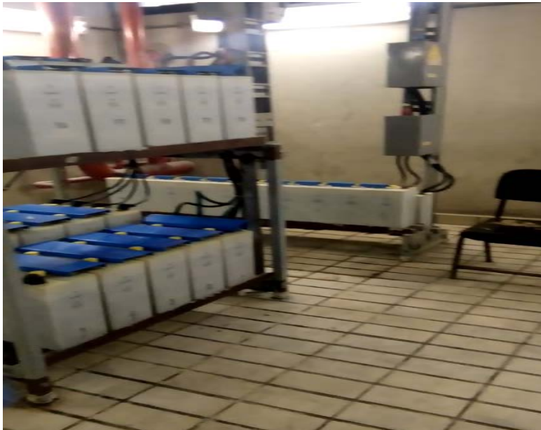
Figure 3.14: Battery Room in Apscl unit-1
