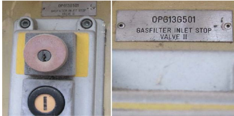
Figure 3.8.1.2: Gas filter inlet shut off valve.
