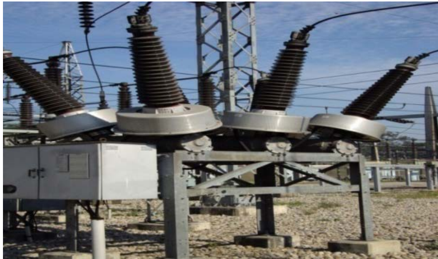
Figure 5.4.1: SF 6 Circuit Breaker used at APSCL Substation
