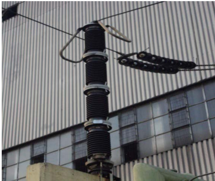
Figure5.6: Lightning arrester in APSCL.
