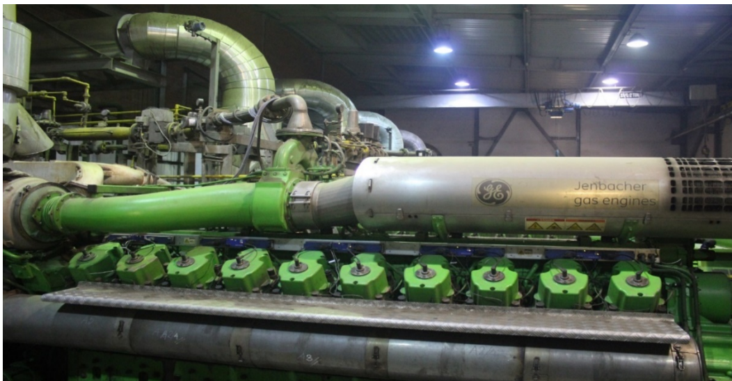
Figure 2.10.1: Jenbacher Gas Engine in APSCL
