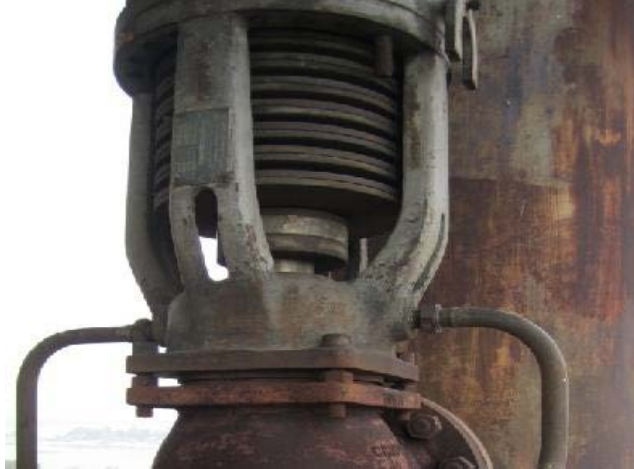
Figure 3.8.7: Super heater safety valve.
