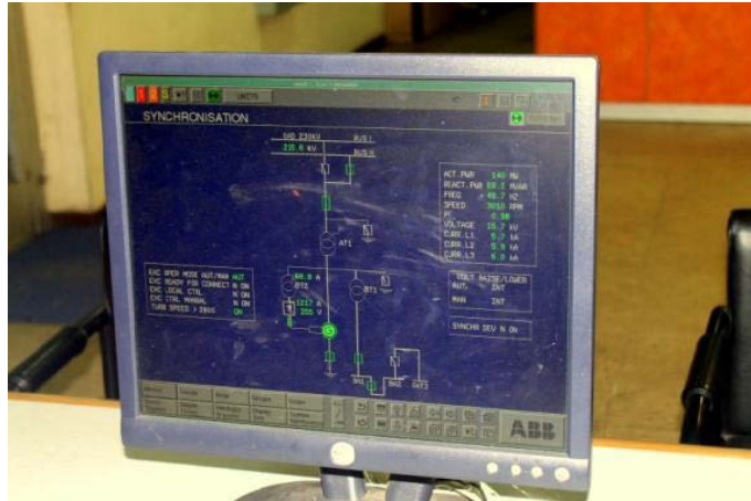
Figure 3.12: Software based control system in 150MW & 11 KV unit 5.
