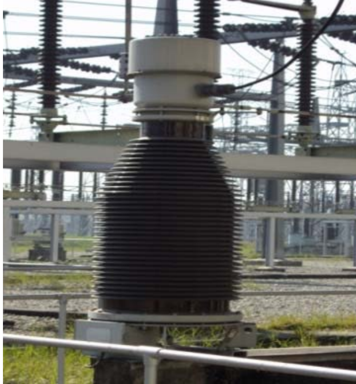
Figure 5.3.2.1 Shows the Current Transformer
