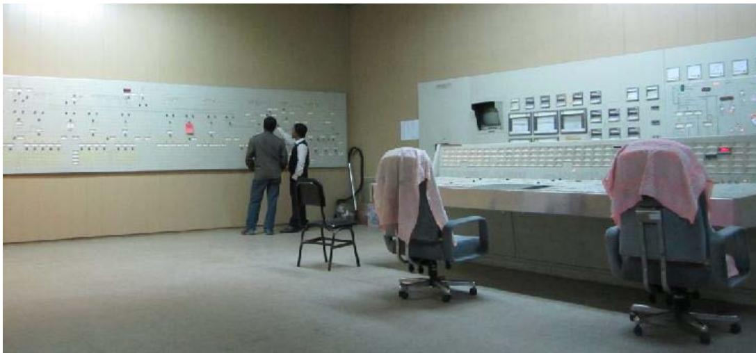
Figure 3.10: Shows the control Room of APSCL
