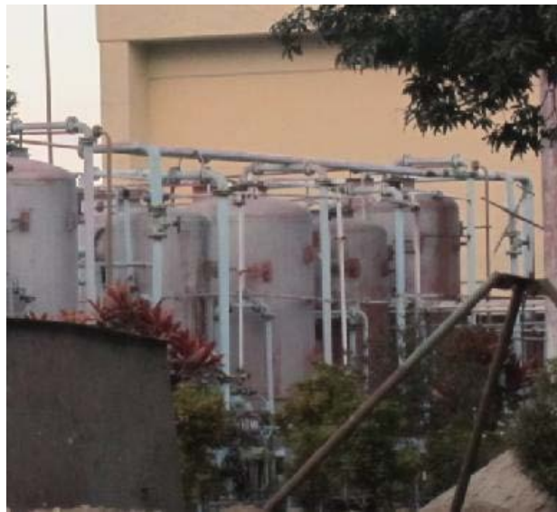
Figure 4.7.2 shows the Hydrogen Plant
