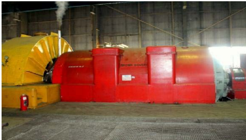
Figure4.3: 150 MW AC generator of unit 3
