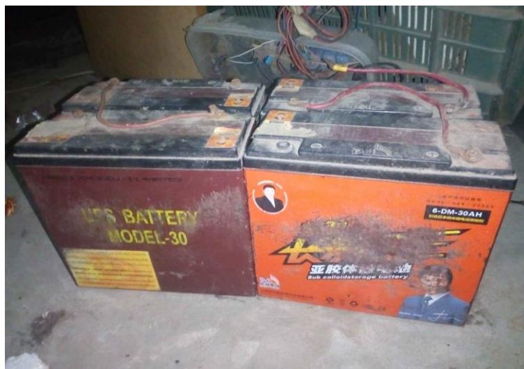
Figure 3.2.1.5: 12v UPS batteries
