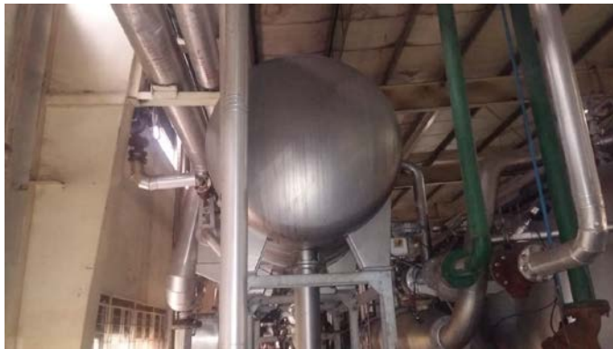
Photo of Reserve Tank.
