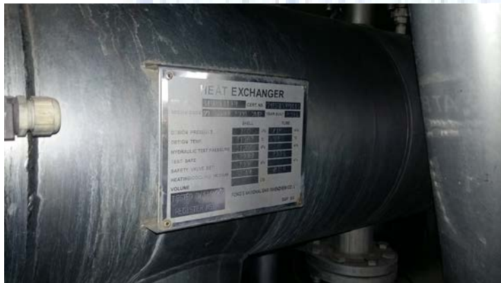
Photo of heat exchanger
