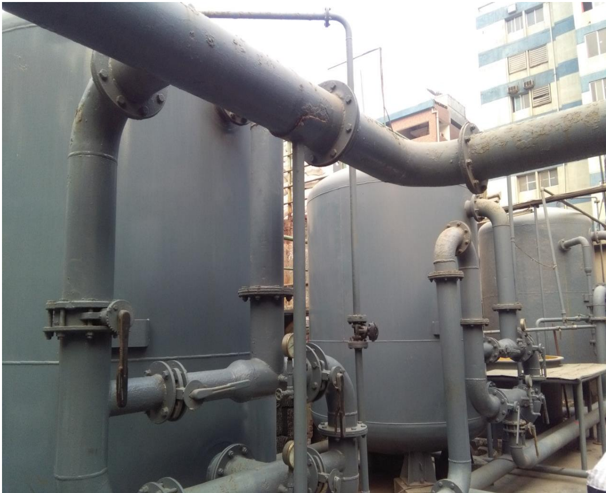
Figure 3. 33: Water Treatment Plant
