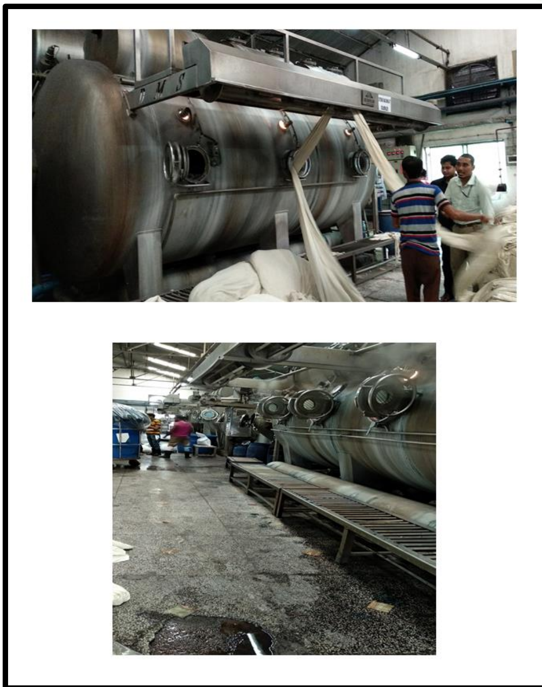
Fig.No:3.10.1 Dyeing section of Montex Fabric ltd .
