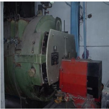
Boiler Gas dryer
