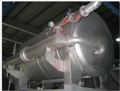
Fig: Reserve Tank
