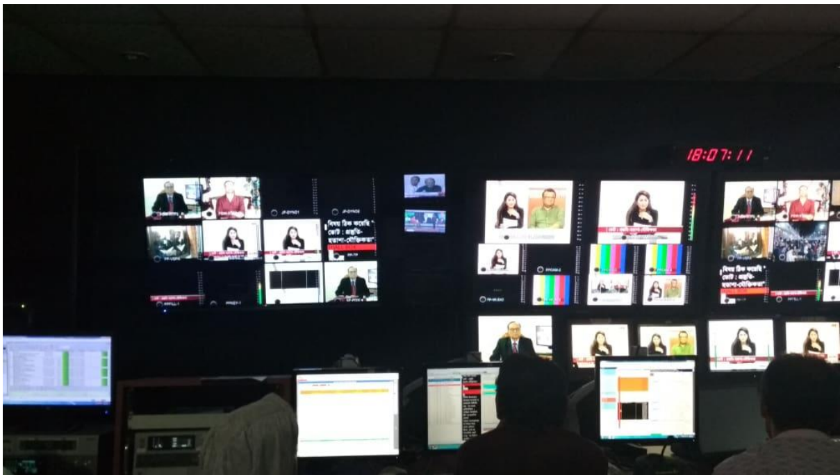
Production Control Room (PCR)
