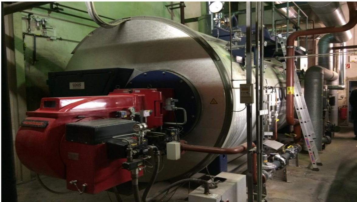
Figure 3.9.2: LOOS strem boiler machine
