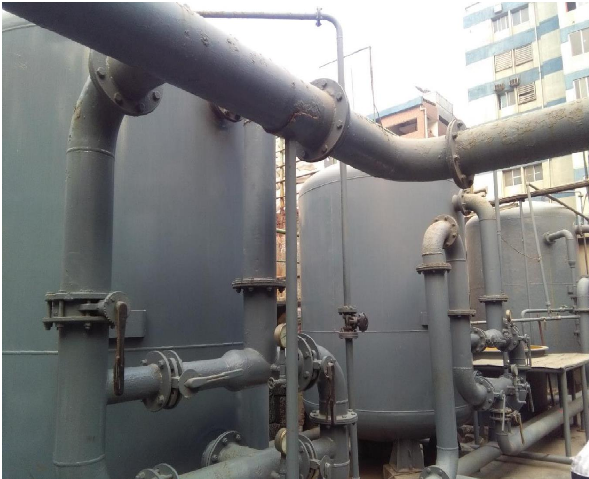
Figure 3.9.1: Water Treatment Plant
