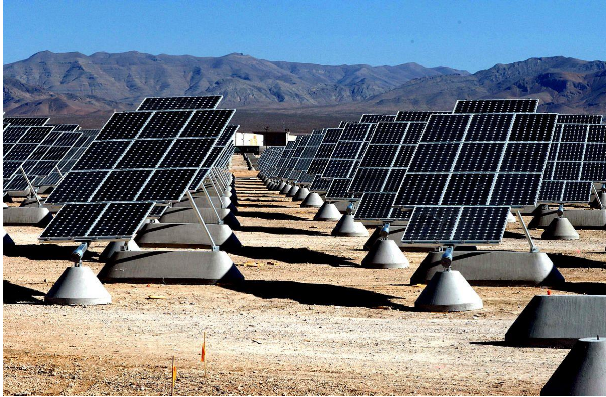
Figure 1.1: Nellis Solar Power Plant, 14 MW power plant installed in North America [6].
