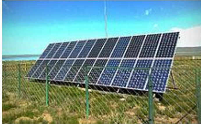
Figure 3.1: A solar array composed of a solar panel with 24 solar modules in rural area.
