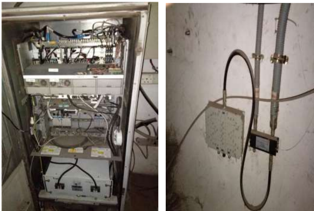
Fig-8.3 - RX Rack with switches & Battery And RRU Connector Board(BTS)
