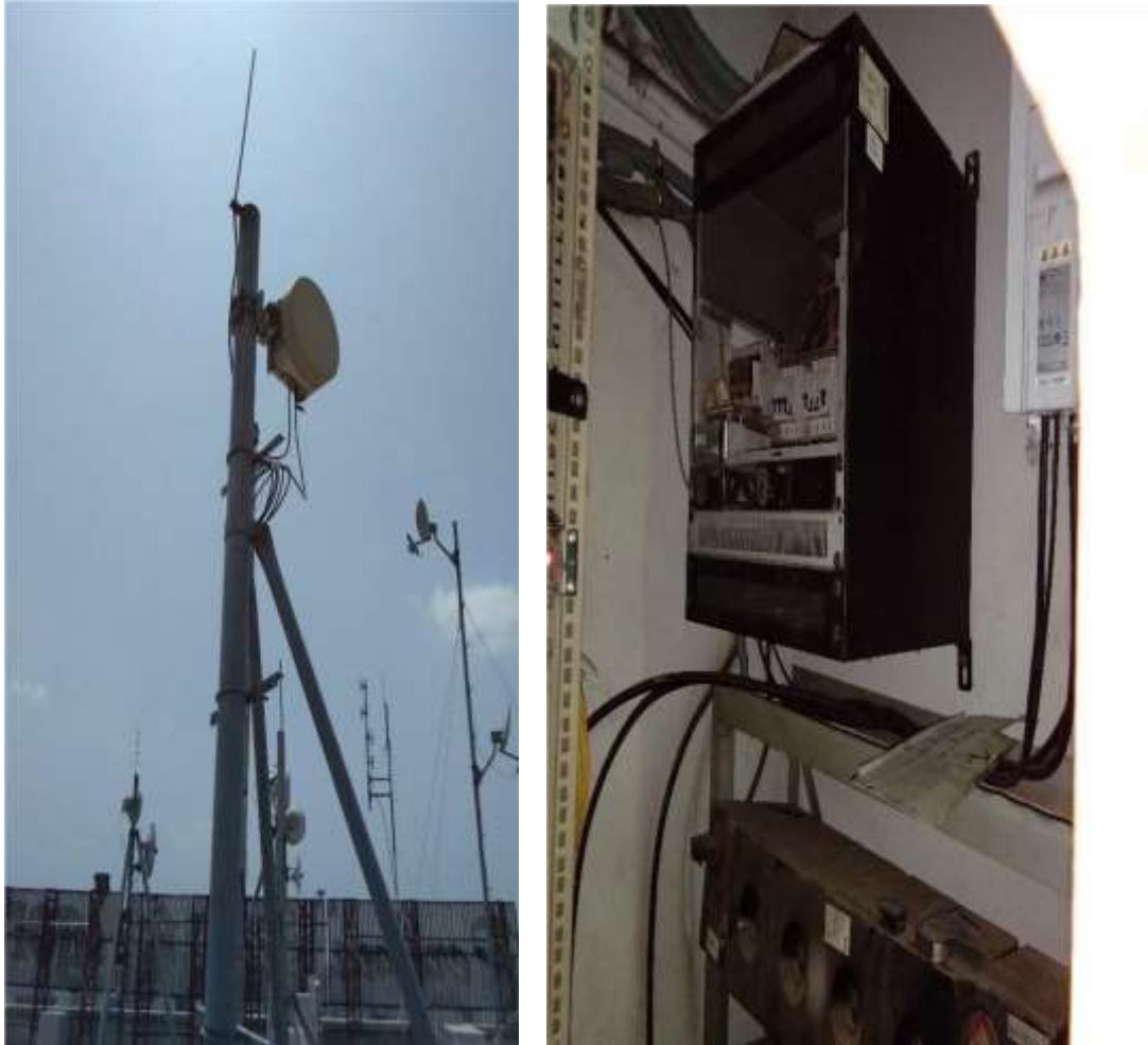
Fig 8.1: ROBI Tower & Switchboard
