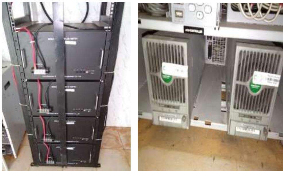
Fig-8.5- BTS site Pictures.(2G & 3G Network) Boards. TXRac .
