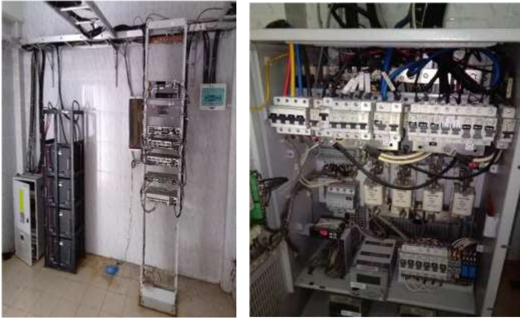
Fig-8.4 Battery with tx rack switch boards
