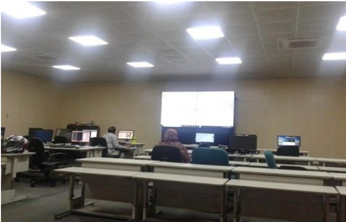
Figure 3.16: BTCL NOC Room
