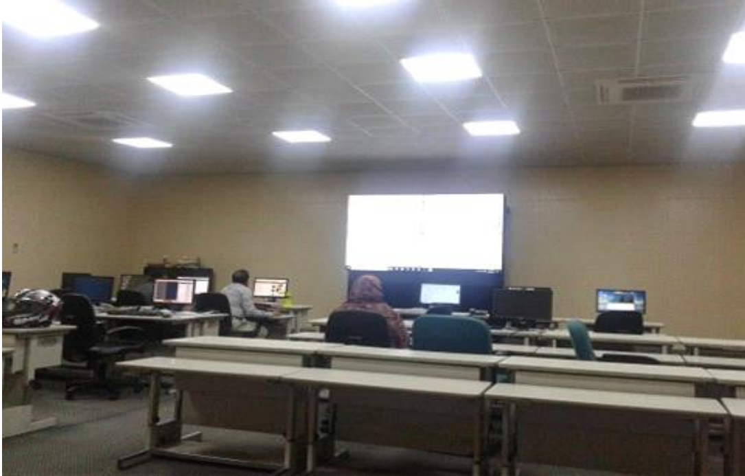
Figure 3.1.17: BTCL NOC Room
