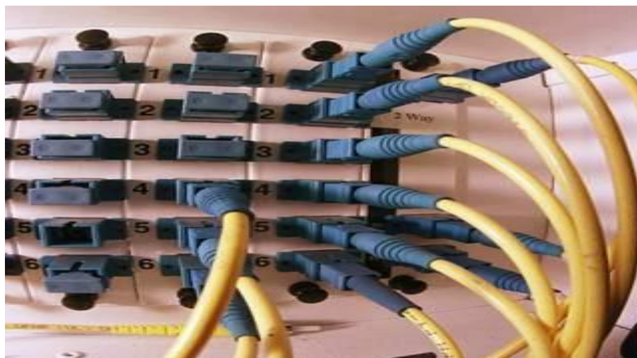
Figure2.1:Cable collection point
