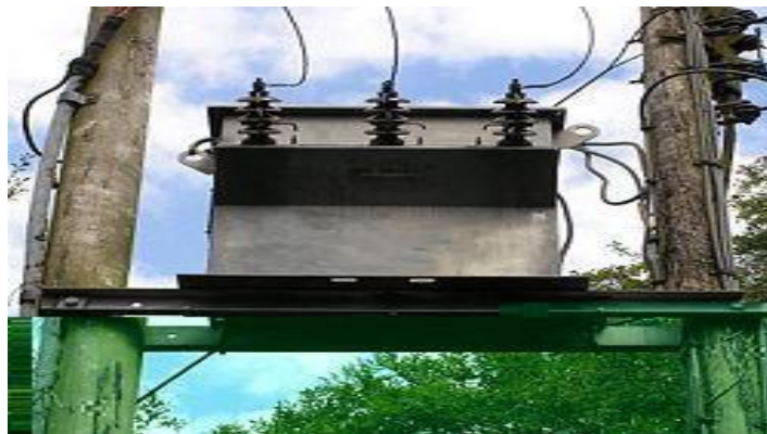
Fig4.1: Three-phase pole-mounted step-down transformer
