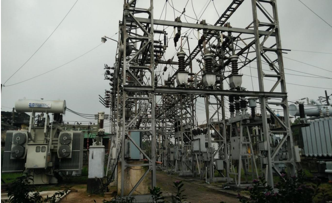
Fig 10.1: Bhurulia dual source 33/11kv indoor substation, Gazipur.
