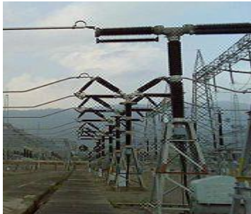
Fig7.8: 400kV SF6 circuit breakers
