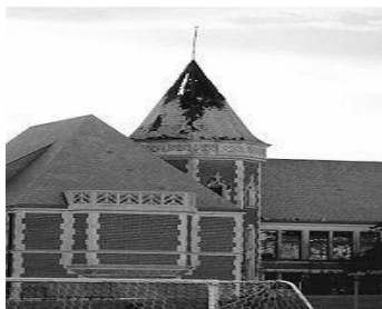
Fig6.2: Example of a grounding system that failed during a lightning strike resulting in a fire.
