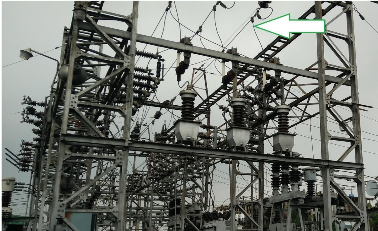
Fig 10.7: 33kv Bus-Bar (marked with arrow)
