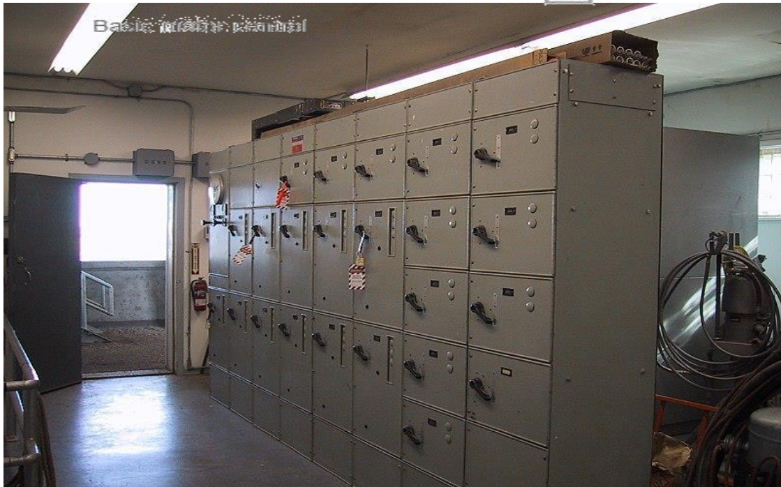
Figure 5.3 Motor panel board
