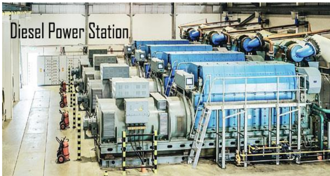
Figure 2.3 Diesel Power Station
