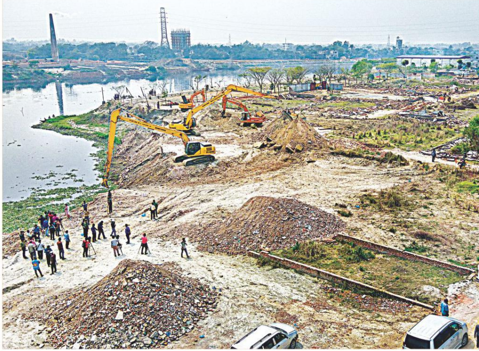
Excavators of Bangladesh Inland Water Transport Authority working on reclaiming a large part of the Buriganga river illegally filled-up by a real estate company in Bosila area of the capital.
