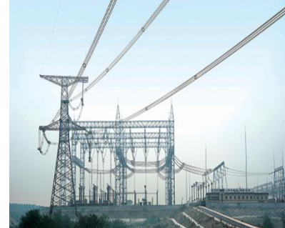
Fig: The smart substation
