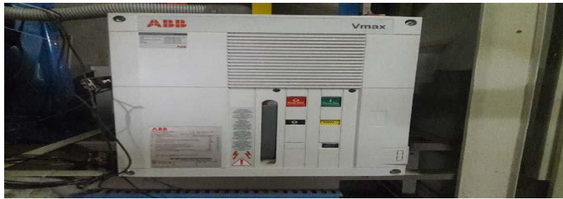
Fig 7.5: Vacuum Circuit Breaker (VCB)
