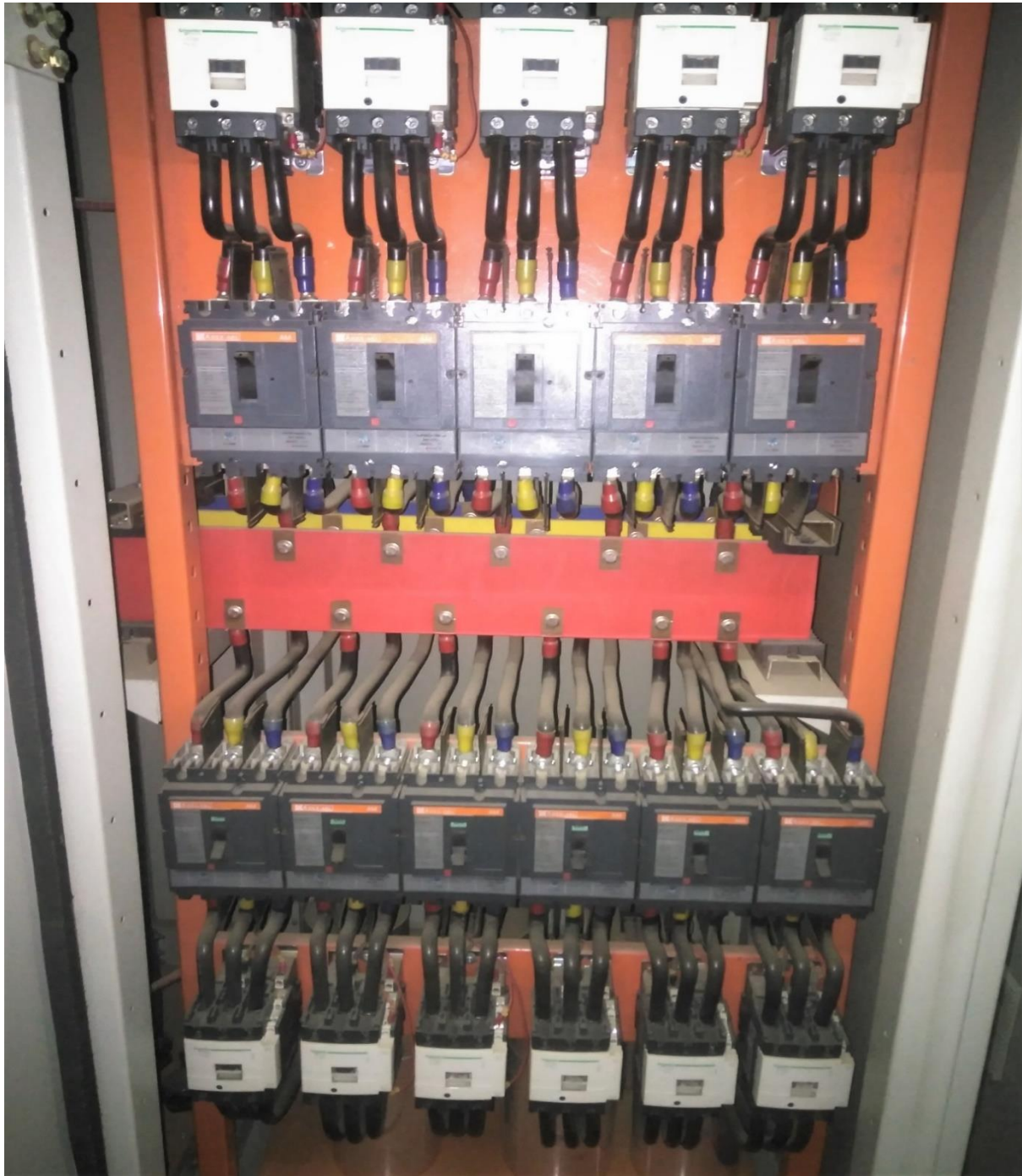
Fig 2.7: Capacitor bank PFI panel
