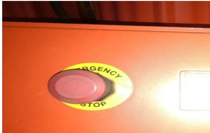
Figure 6.1: Emergency Stop Button in generator
