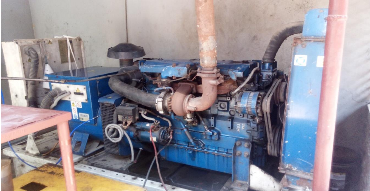
Fig 2.8: Diesel generator for backup
