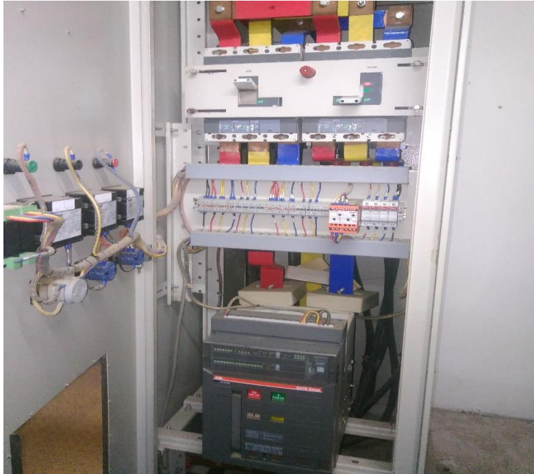
Figure 2.4: Switchgear of Substation
