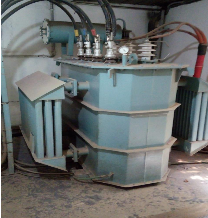
Figure 4.1: Distribution Transformer in BHDP
