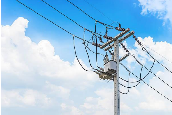
Figure: 3.8-Electric pole with capacitor
