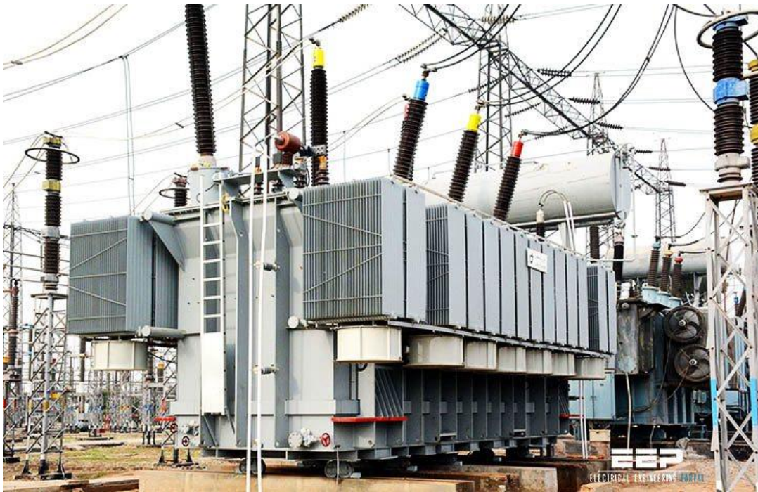
Figure: 5.6-Substation of transformer
