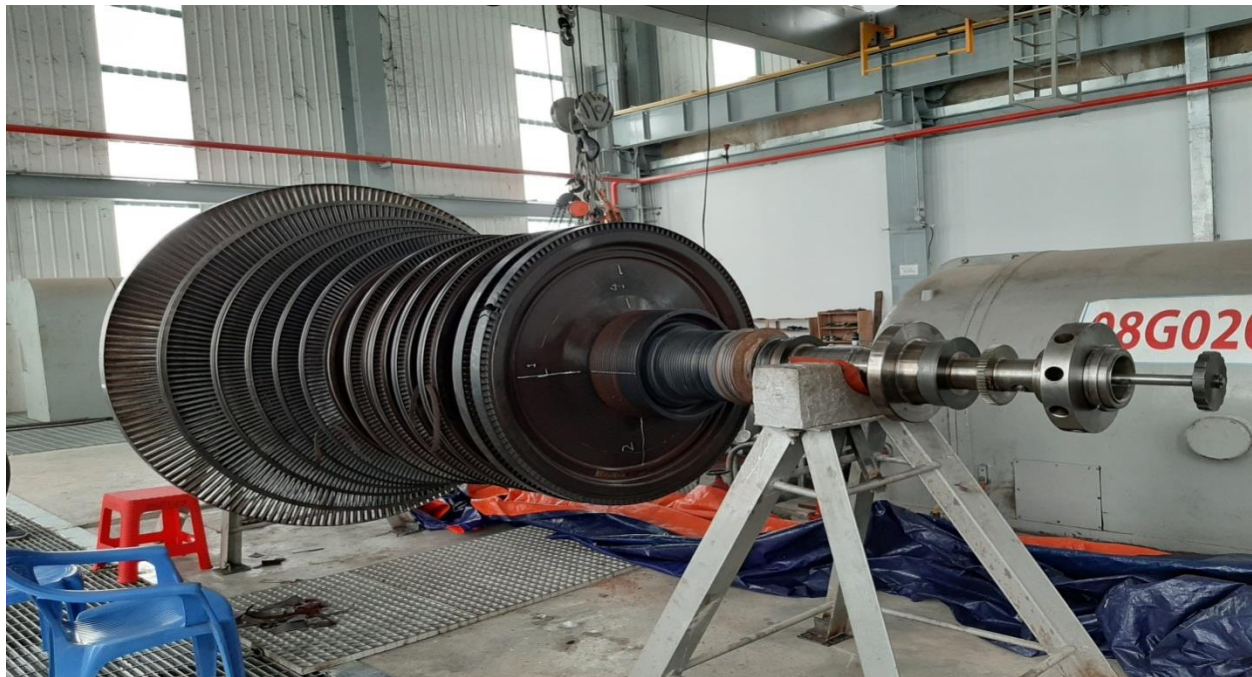
Fig3.5: The rotor of turbine is connected by coupling with rotor of generator.
