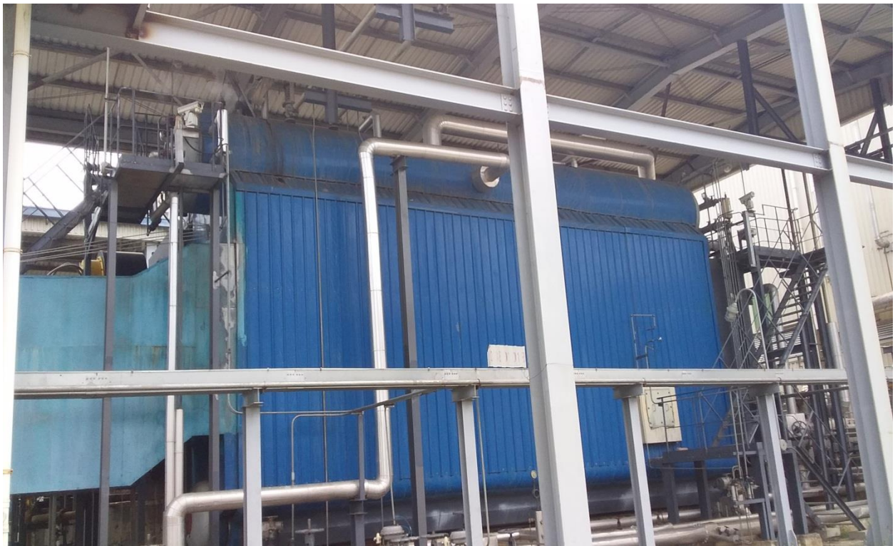
Fig3.2: Boiler of SFCL.
