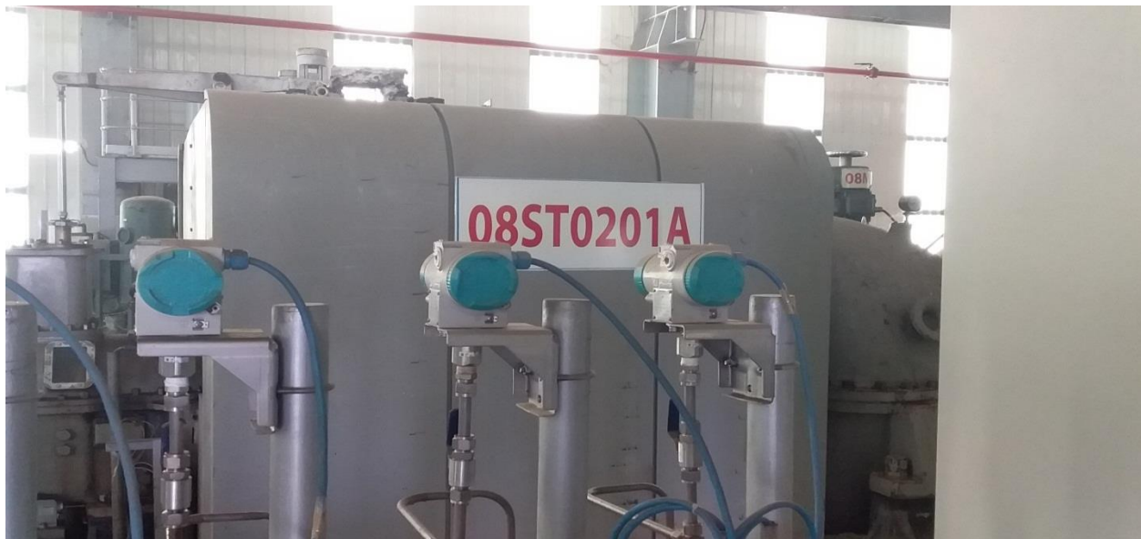
Fig 3.3: Steam Turbine Of SFCL.
