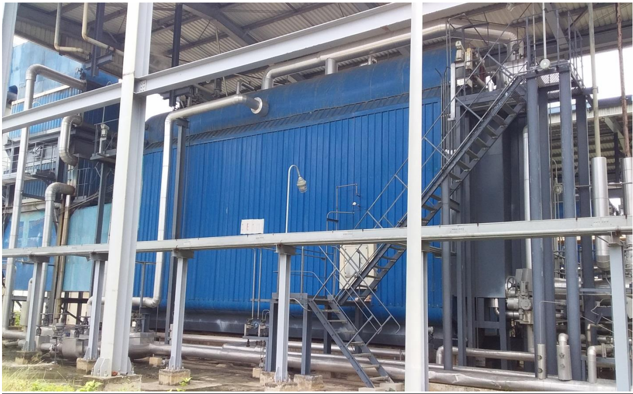
Fig3.1: Boiler of SFCL.
