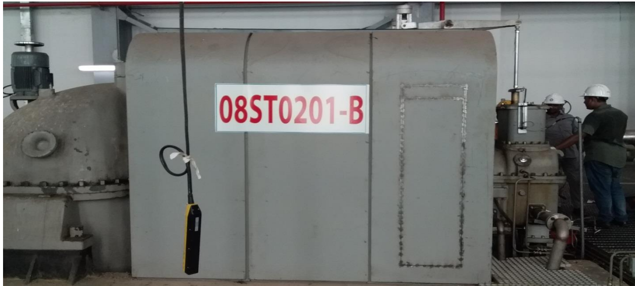
Fig3.4: Steam Turbine Of SFCL.
