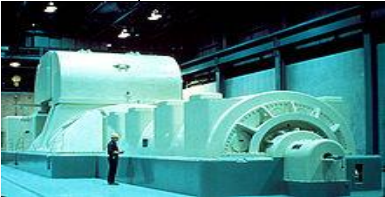
A modern steam turbine generator installation
