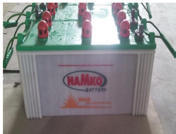
Figure 3.15: Battery regularly maintained
