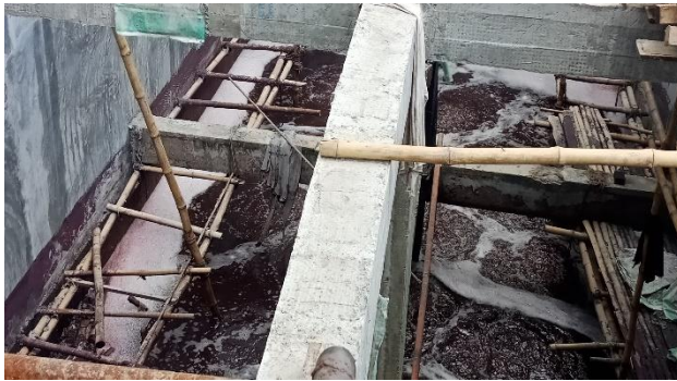
Figure : Screening Unit
