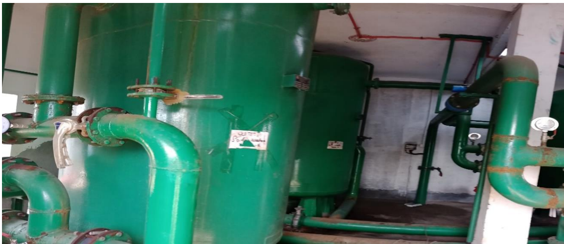
Figure: Water Treatment Plane
