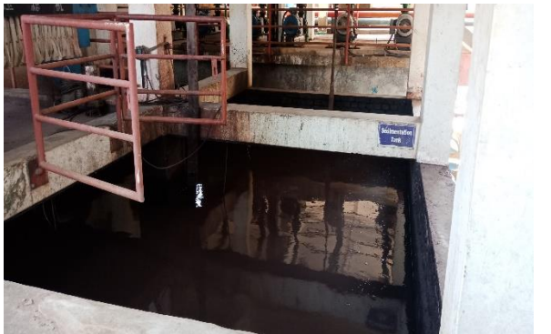
Figure : Sedimentation Tank
