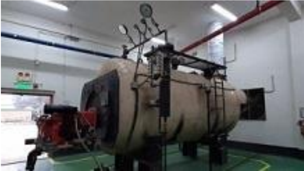
Picture of boiler
