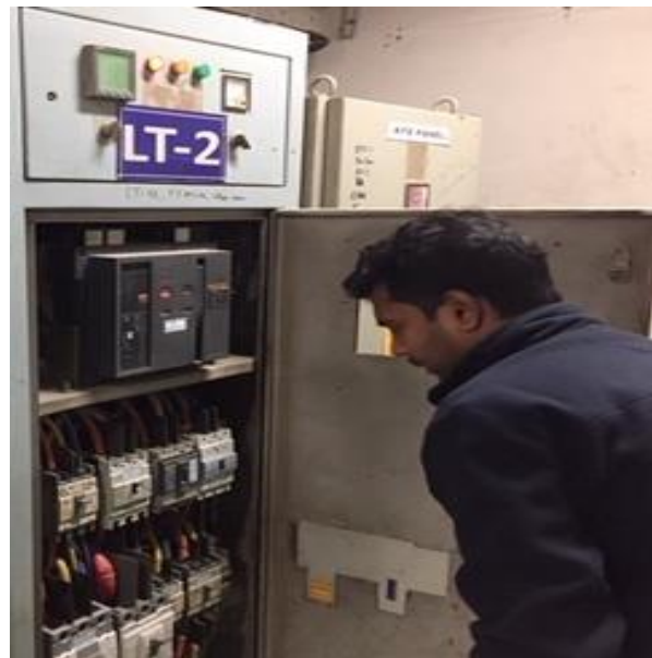
Figure:LT panel of substation
