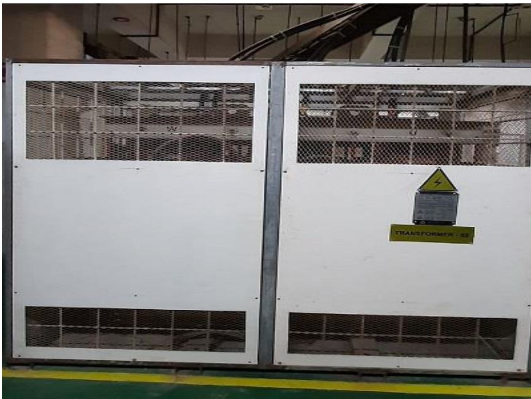
Physical picture of transformer:
