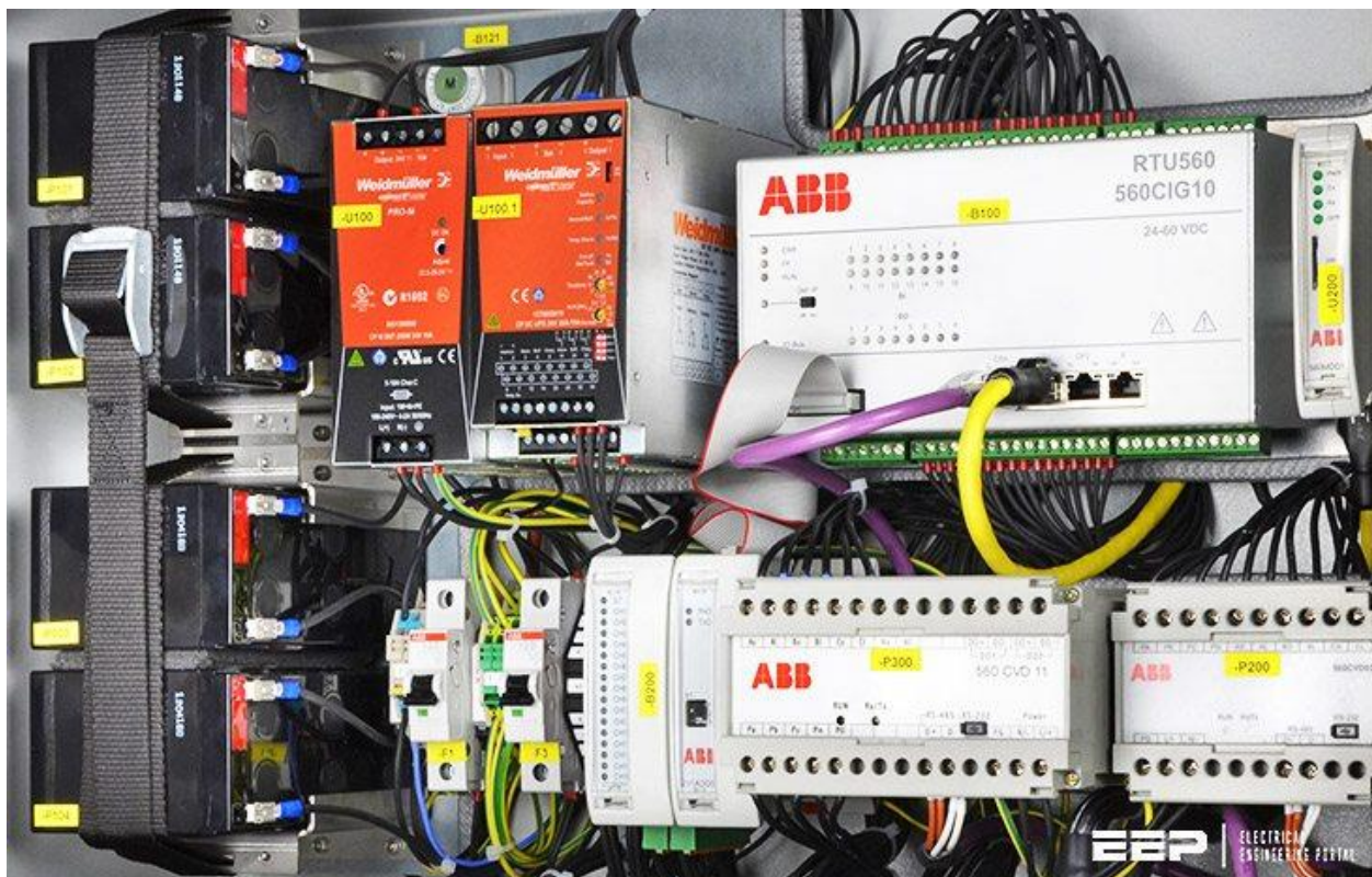
Fig: 4.2- PLC Control Board
