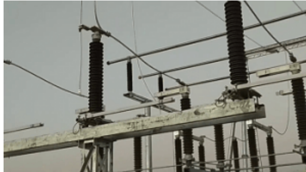
Fig 3.14: Bus bar in Sub-station
