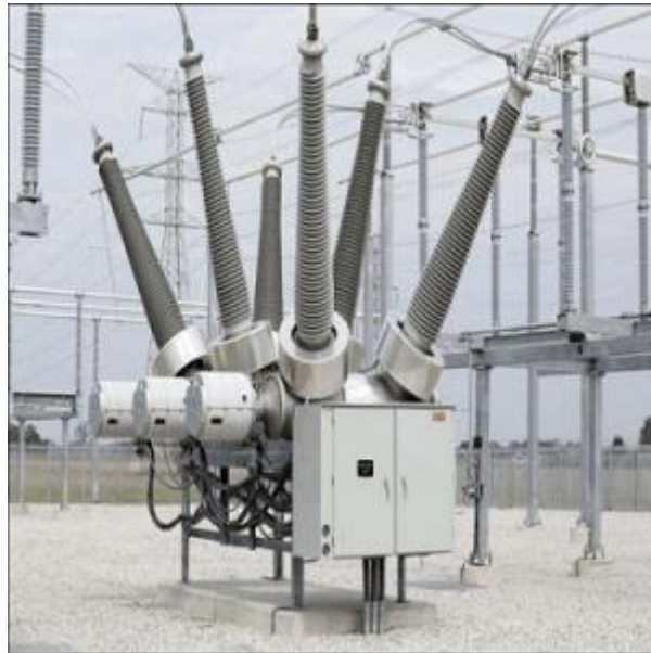
Fig 3.13: Circuit Breaker in Substation
