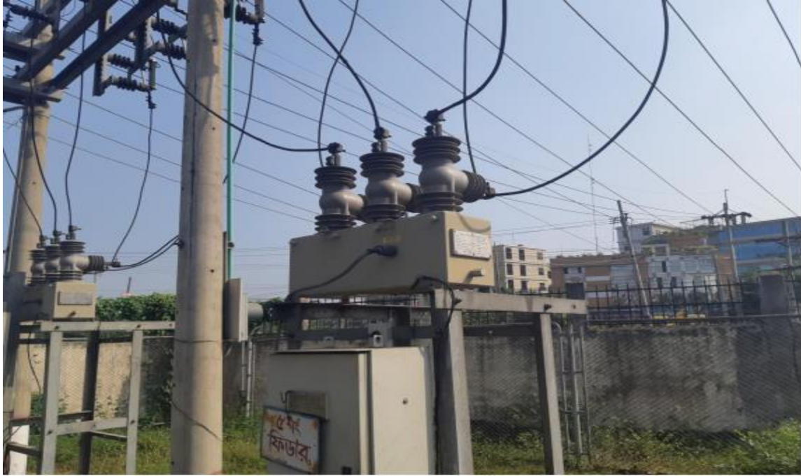
Figure 5.7: Feeding system of transformer in sub-station
