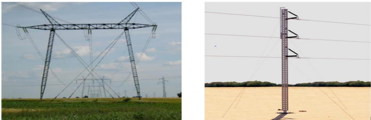
Fig:4.4 Sample of Guyed OHTL support
