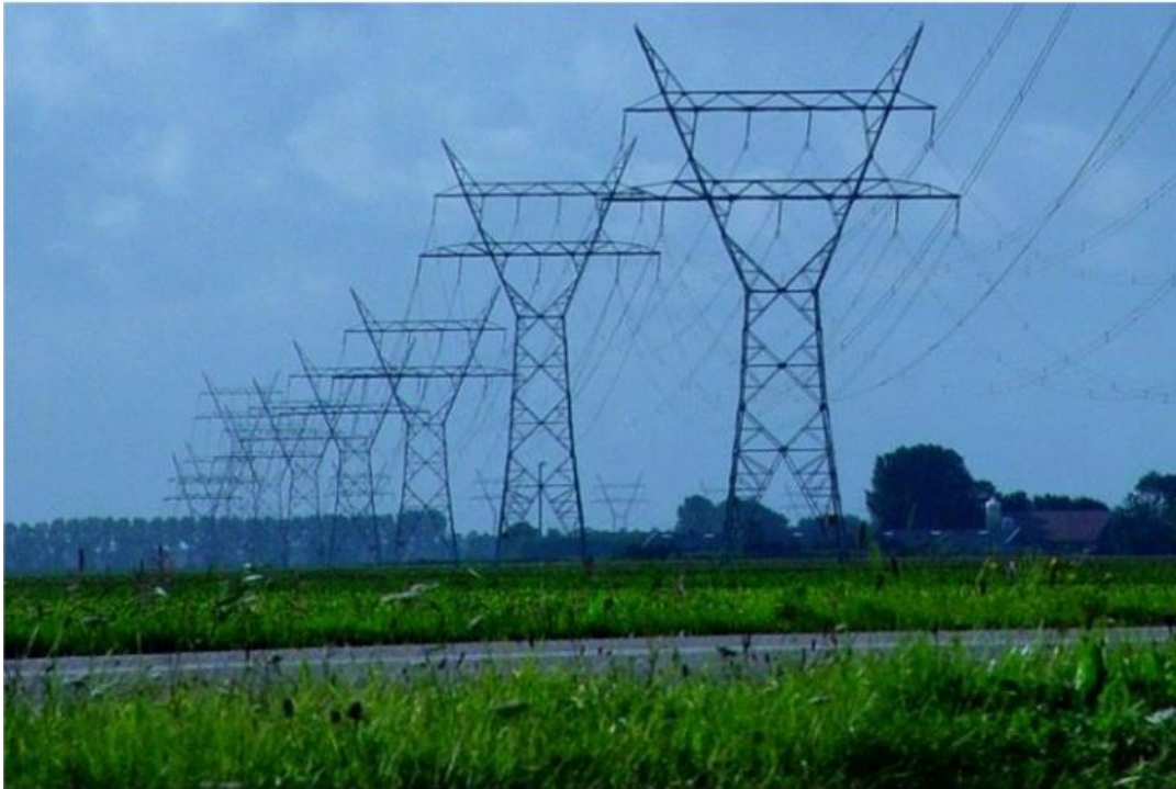
Fig:4.1 Overhead transmission line
