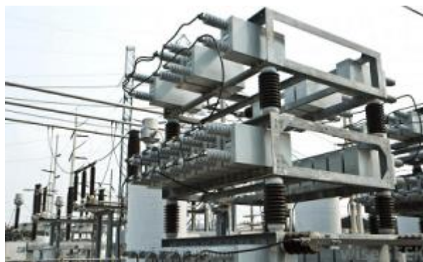
Fig 3.17: Capacitor Bank in Substation
