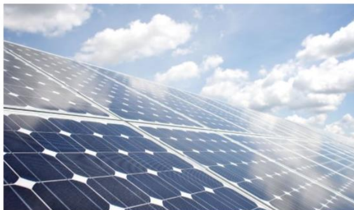
Power plant - Photovoltaic
