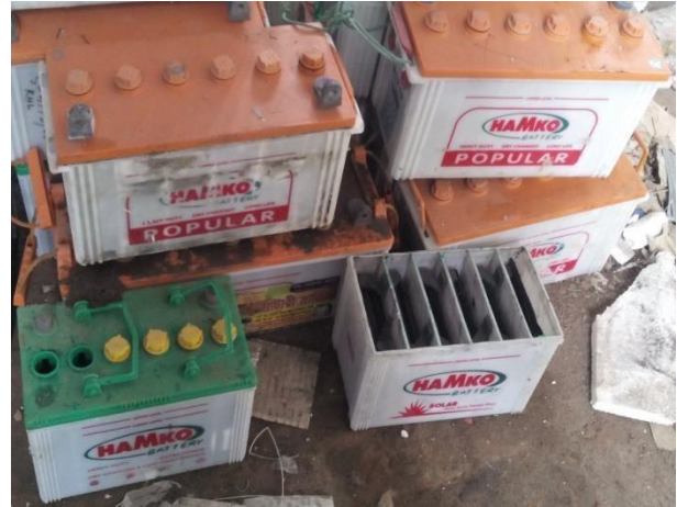
Figure 3.16: Wasted batteries due to lack of maintenance
