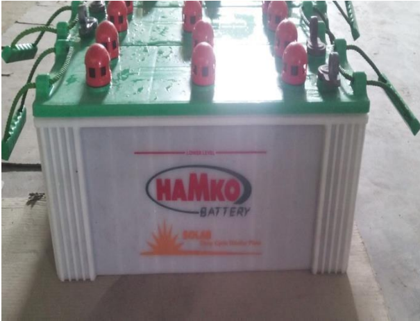
Figure 3.15: Battery regularly maintained
