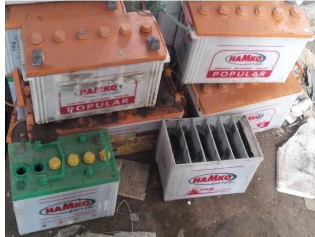
Figure 3.16: Wasted batteries due to lack of maintenance
