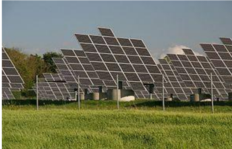
Figure 3-2: PV farm or solar park
