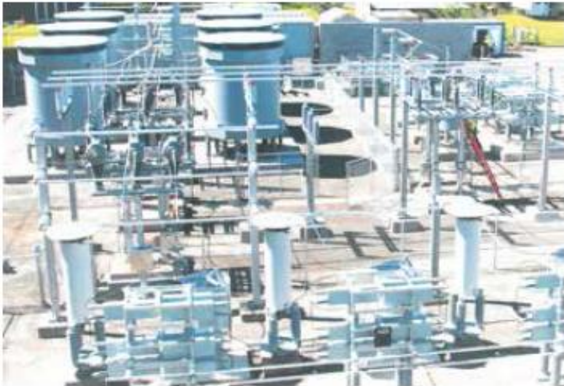
Directly connected SVC
