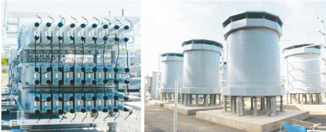
Fig. 4.4: Shunt capacitors and reactors
