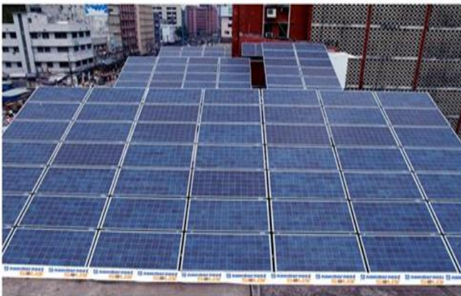
Fig 4.5.4b: Rooftop solar system on the roof of Wapda building.
