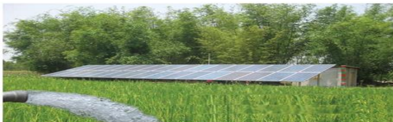
Figure4.5.6b: Solar Irrigation project SHIKAPUR, PANCHAGAR
