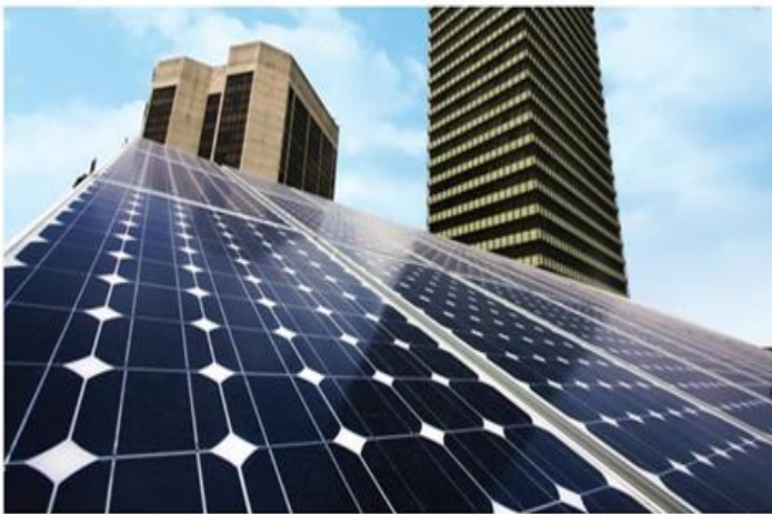
Fig 4.5.4.a: Rooftop solar system on the roof of Bangladesh Bank
