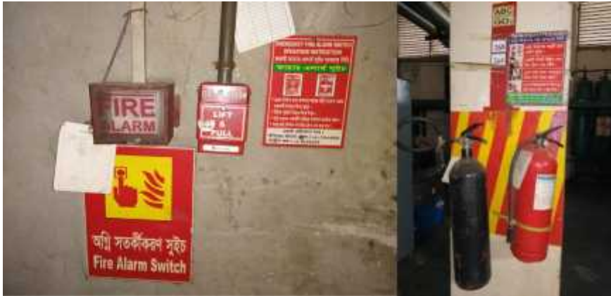
Figure 5.1: CO 2 fire safety cylinders for internal instrument protection in Liz Fashion Industry
