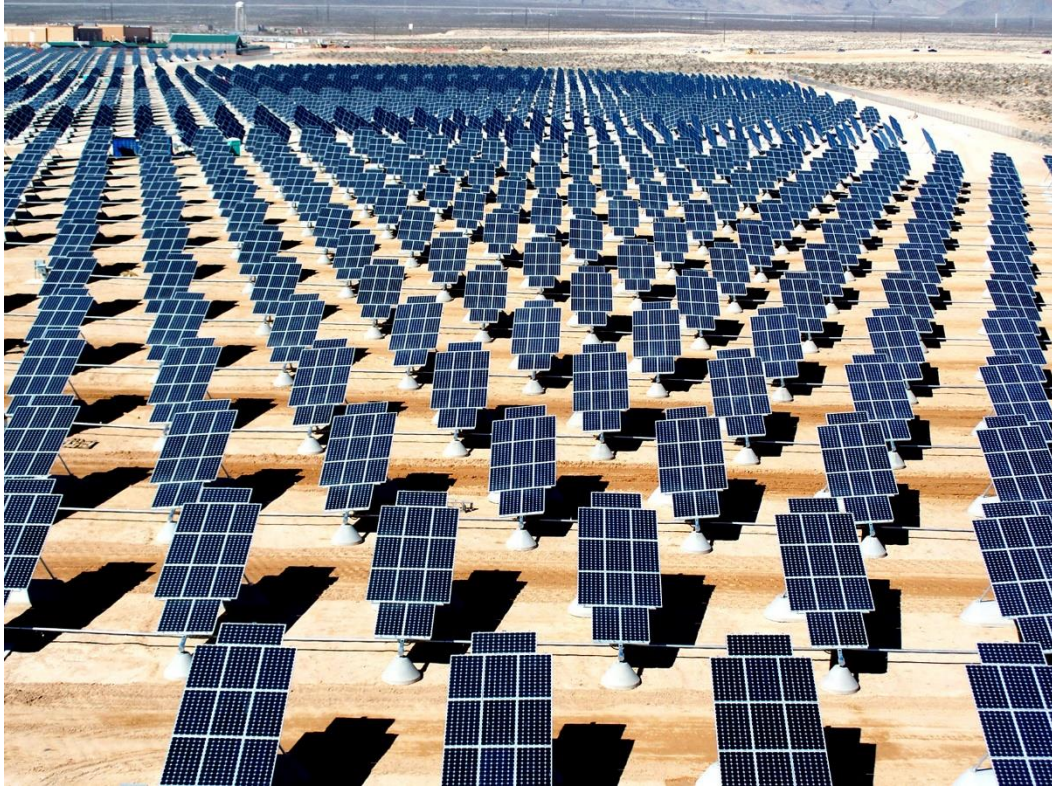
Figure 2.2: Photovoltaic Power Station
