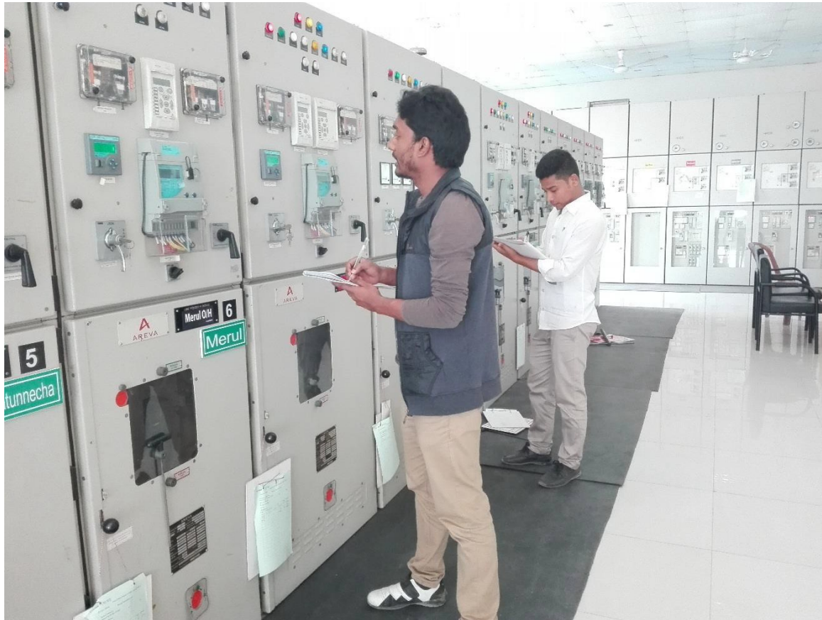
Figure 5.7: Control room at substation
