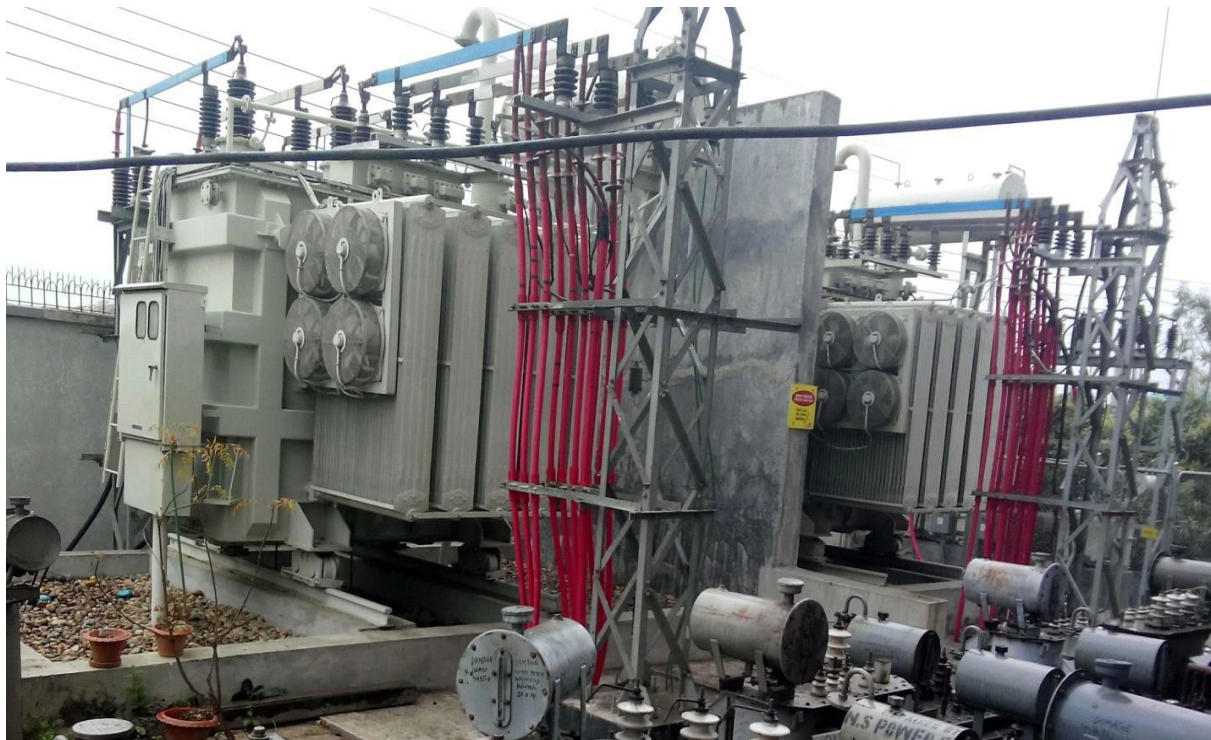
Figure 3.3: Power Transformer T4 & T5
