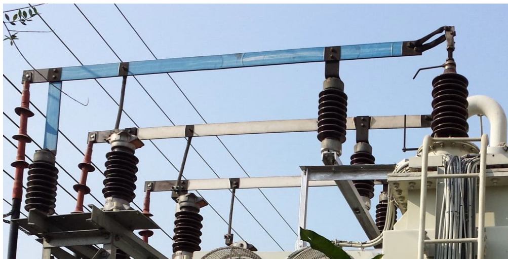
Figure 3.2: 132KV incoming source from Uttara Grid, CT, L.A, PT, HT Bushing
