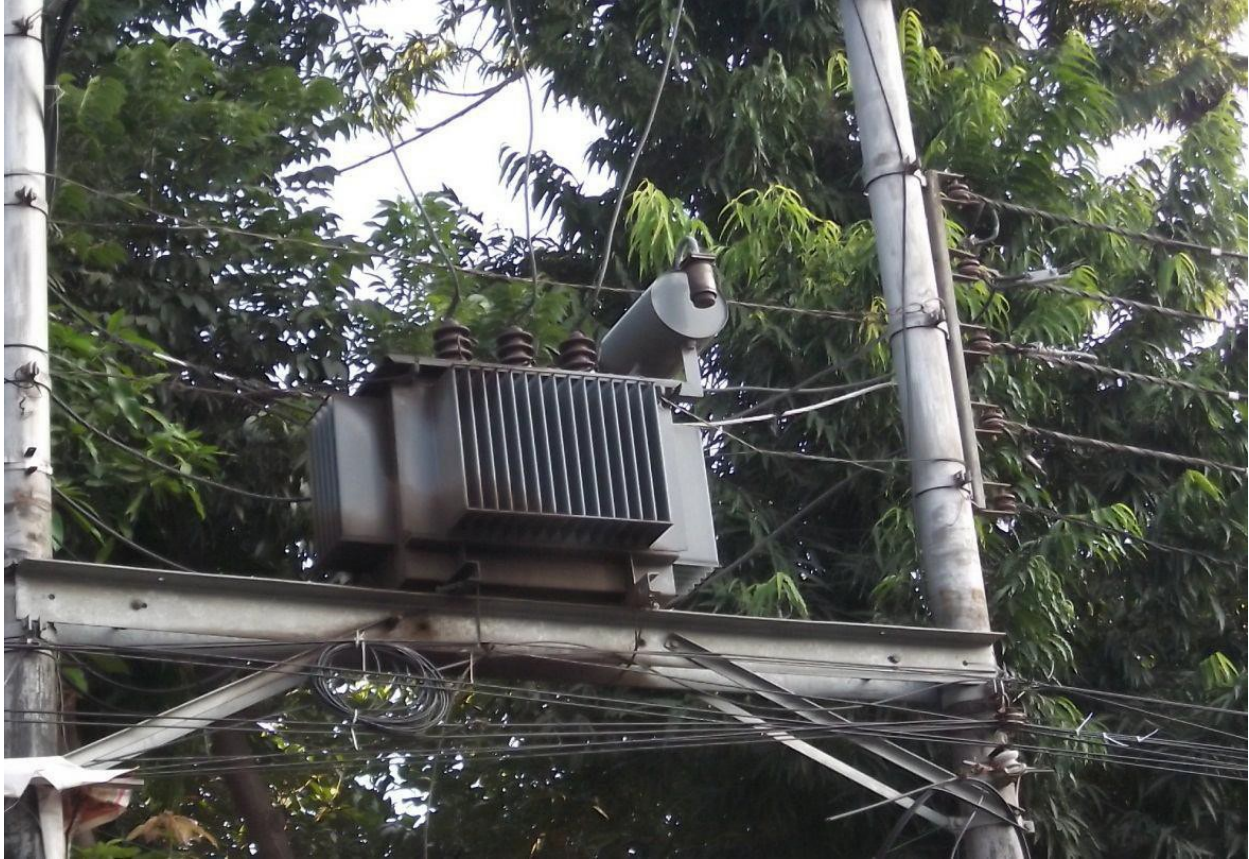
Figure 5.5: The 11KV/440KV distribution transformer.
