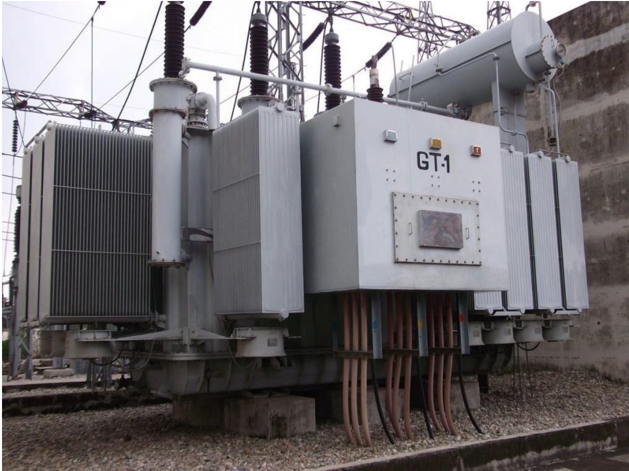
Figure 4.1: 132/33 KV Power transformer (GT1) at Digun Sub-station.
