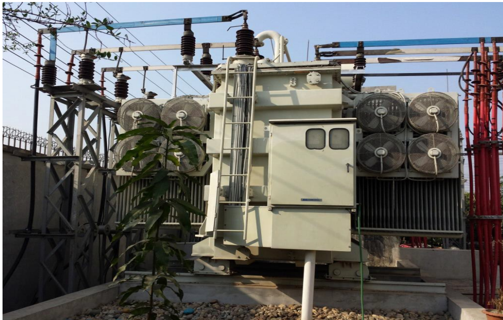
Figure 3.1: Power Transformer (132/33) at Digun Substation
