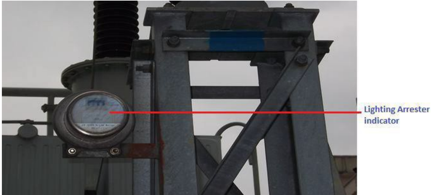
Figure 4.12: Lighting arrester indicator at Digun grid-substation.
