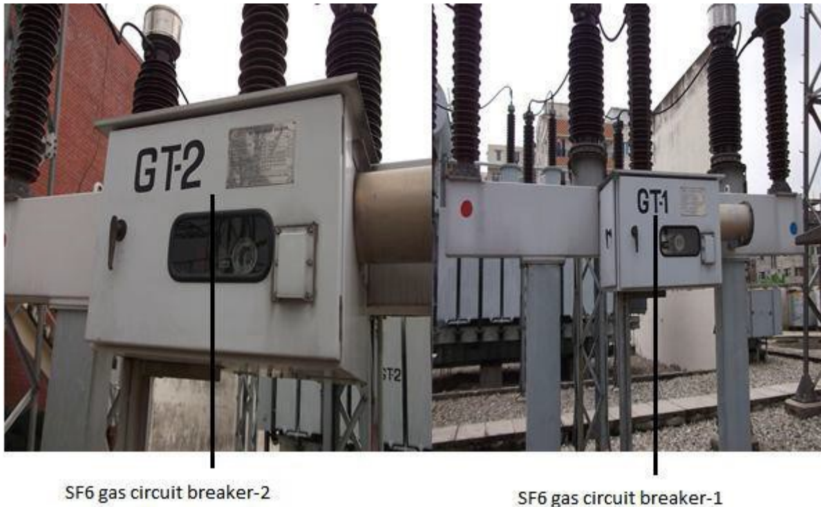
Figure 4.8: SF6 gas circuit breaker at Digun grid-substation.
