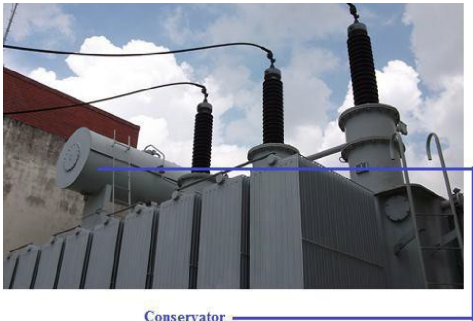
Figure 4.3: Conservator tank at Digun Substation.
