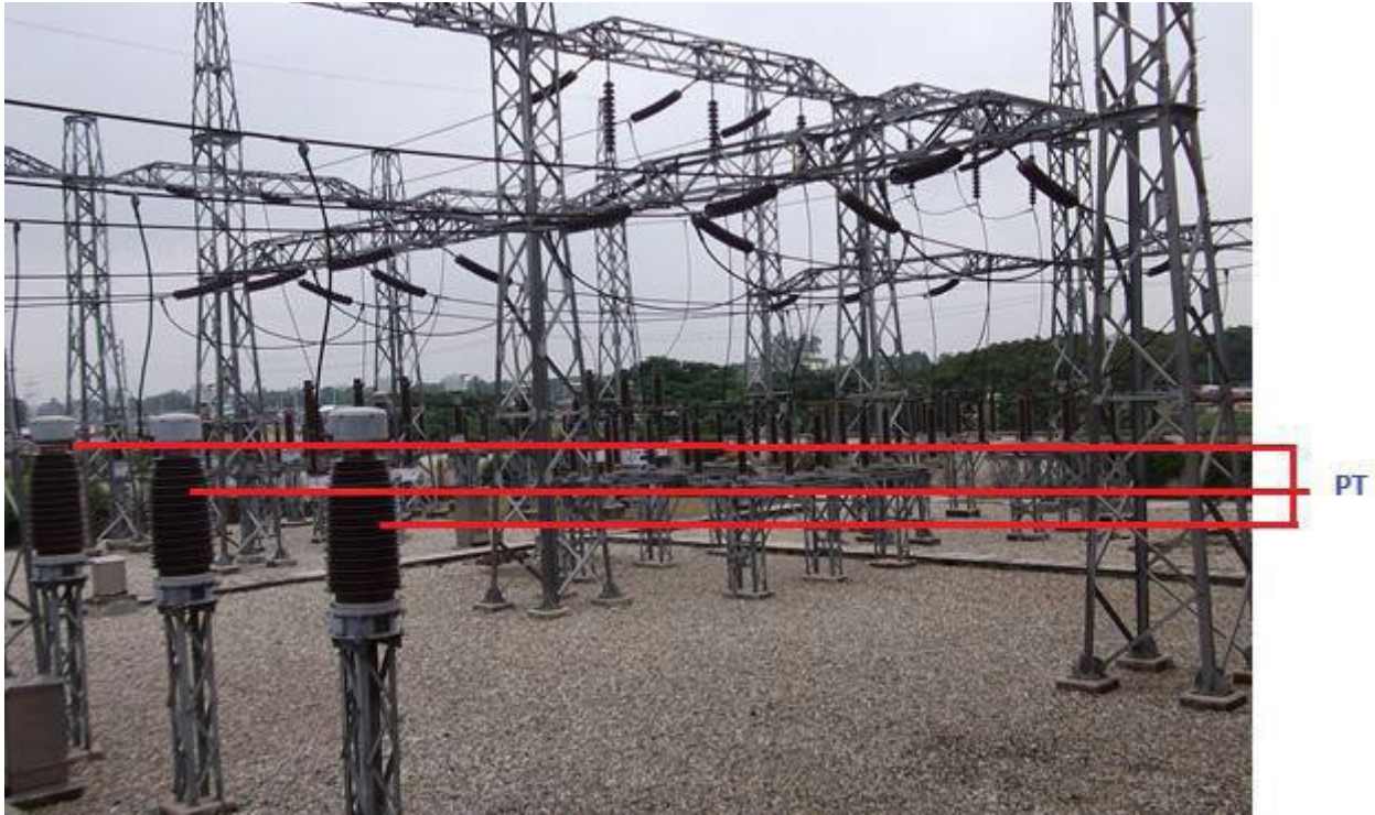
Figure 4.9: Potential transformer at Digun grid-substation.
