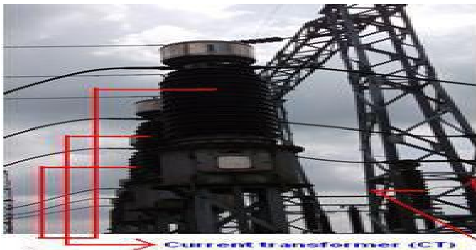
Figure 4.10: Current transformer at Digun grid-substation.
