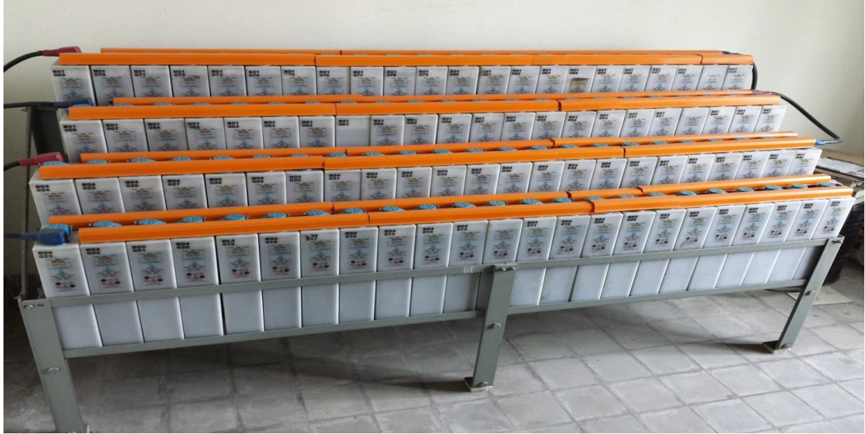
Figure 4.14: Battery backup system of 132/33/11KV Digun grid-substation.
