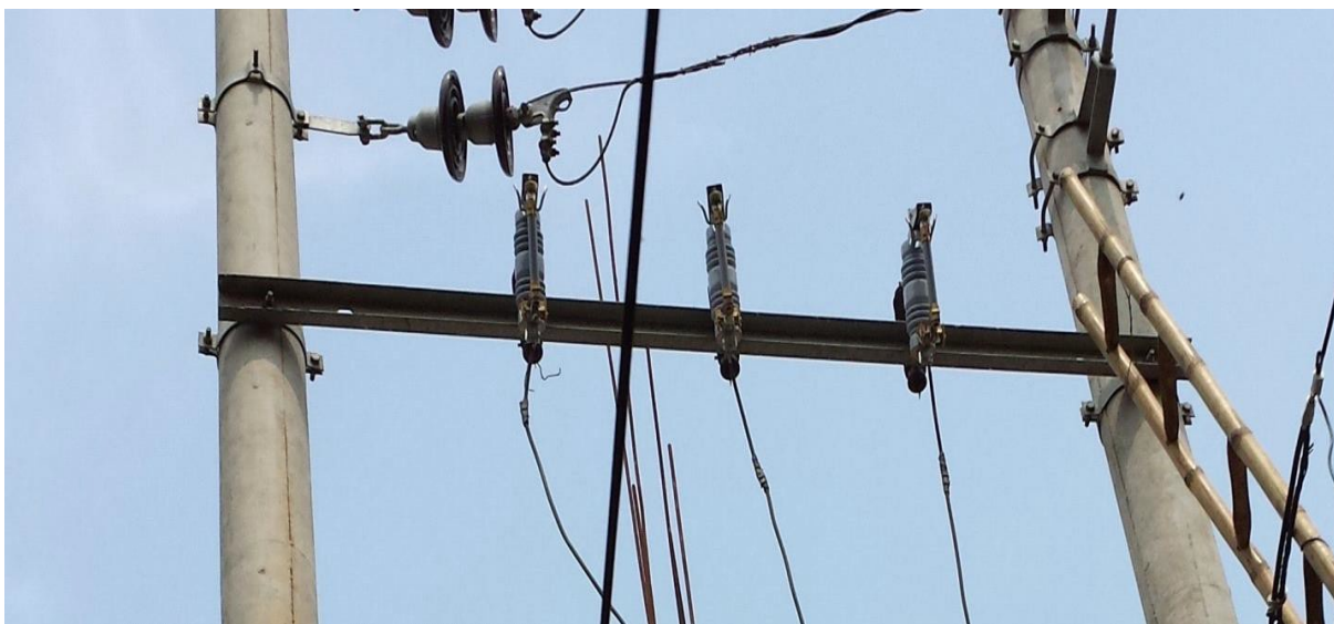
Figure 5.6: Drop out Fuse under Digun Feeder.
