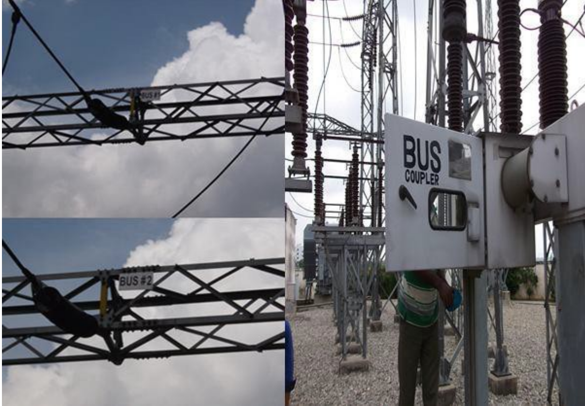
Figure 4.13: 132 KV bus bars and bus coupler at Digun grid-substation.
