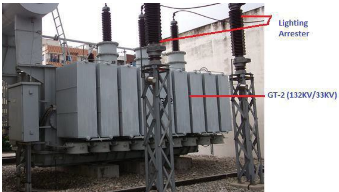
Figure 4.11: Lighting Arrester and GT-2 at Digun grid-substation.
