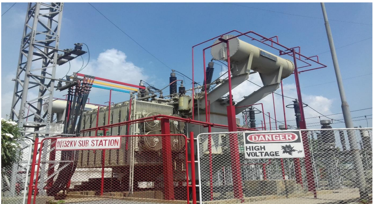
Figure 4.3: (11/132) KV Power Transformer
