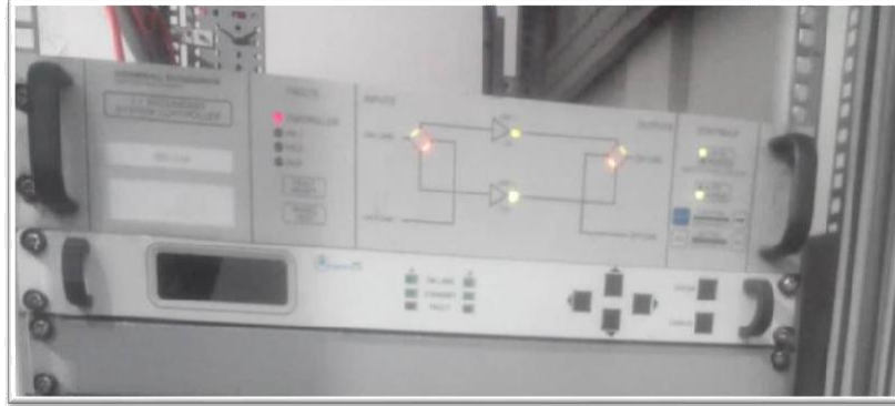
Figure 3.7– Earth Station System Controller
