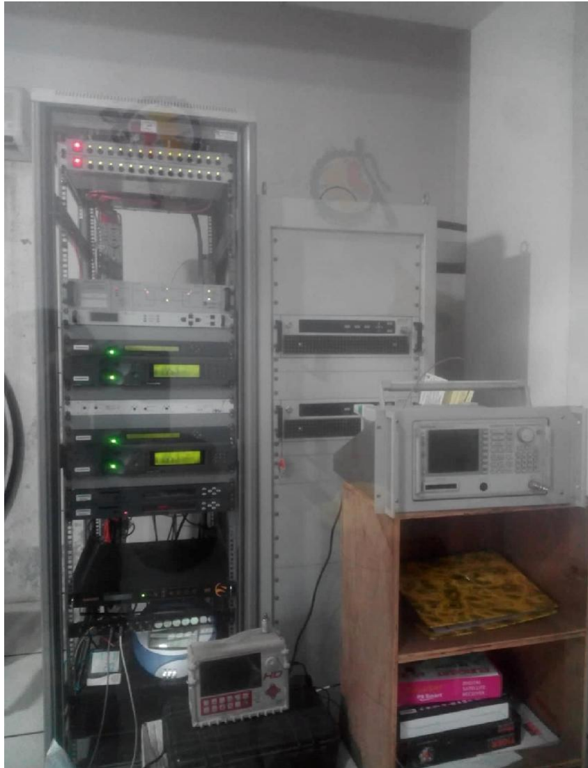
Figure 3.4 - SOMOY TV Earth Station Equipment
