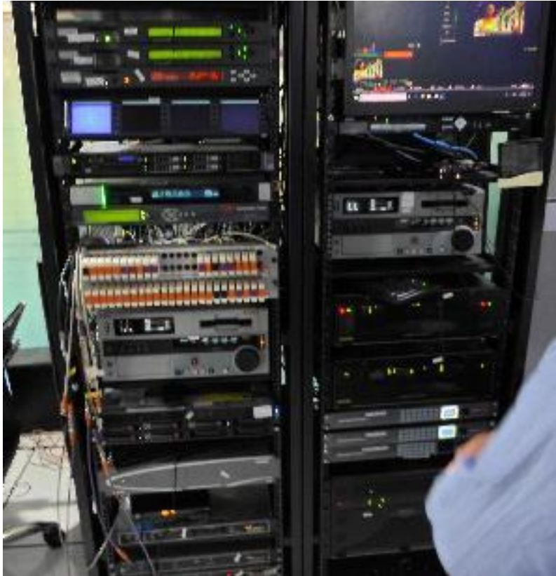
Figure 2.5- INGEST Room Rack and Machines
