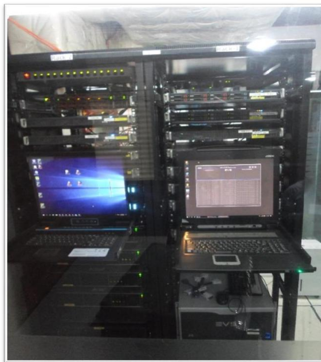
Figure 2.20 –Central Equipment Room
