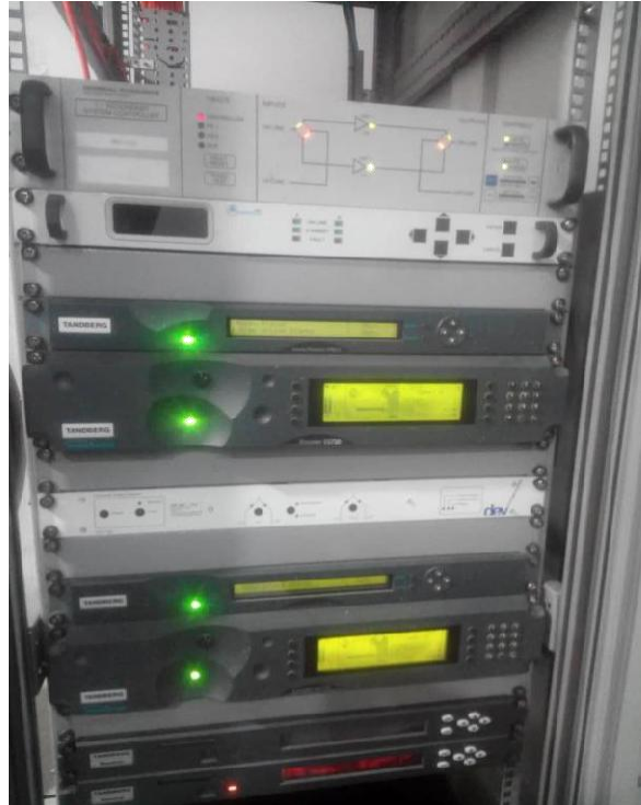
Figure 3.9- Up Converter Main & Back Up
