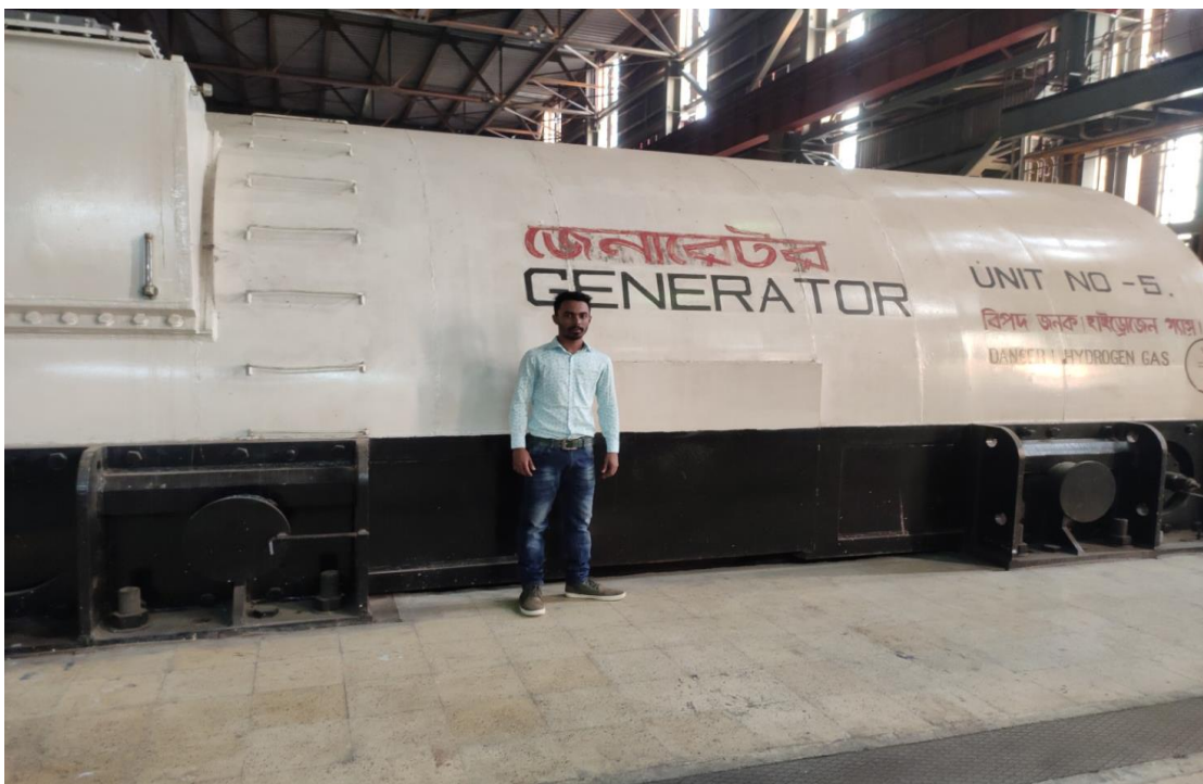
Fig 7.3: 210 MW Generator in GPS
