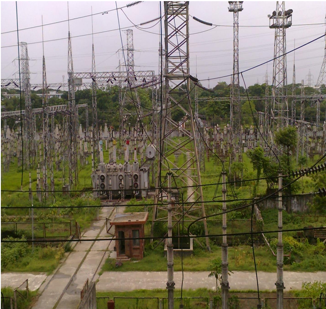
Fig 2.3: Substations of GPS.
