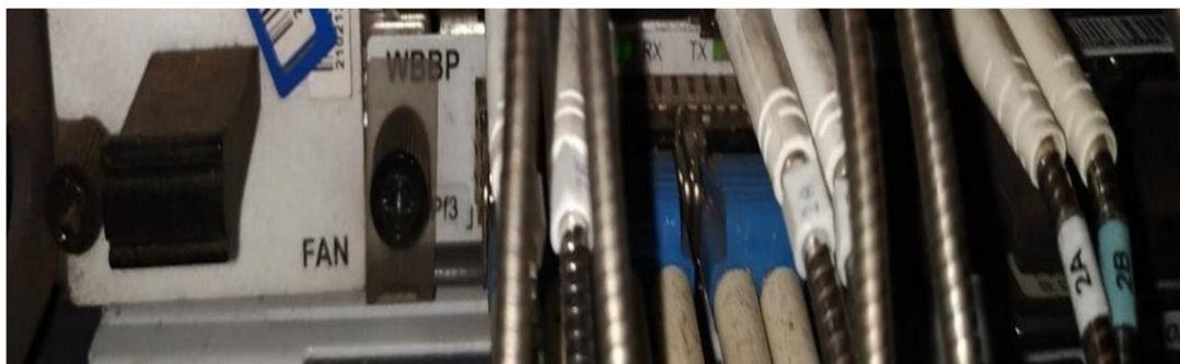
Fig-4.9: WCDMA baseband processing unit Function:
