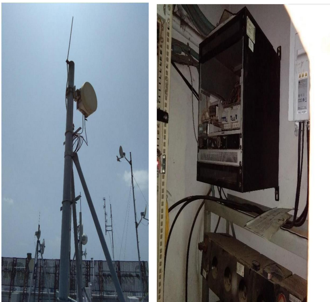
Fig 6.1: ROBI Tower & Switchboard
