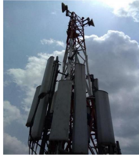
Fig-2.2: Airtel 3G Tower & Switchboard
