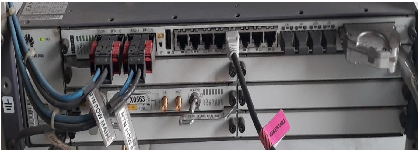
DCDU (Direct Current Distribution Unit)
