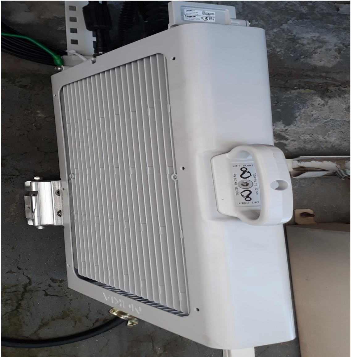
Fig-5.11: RRU Picture in site
