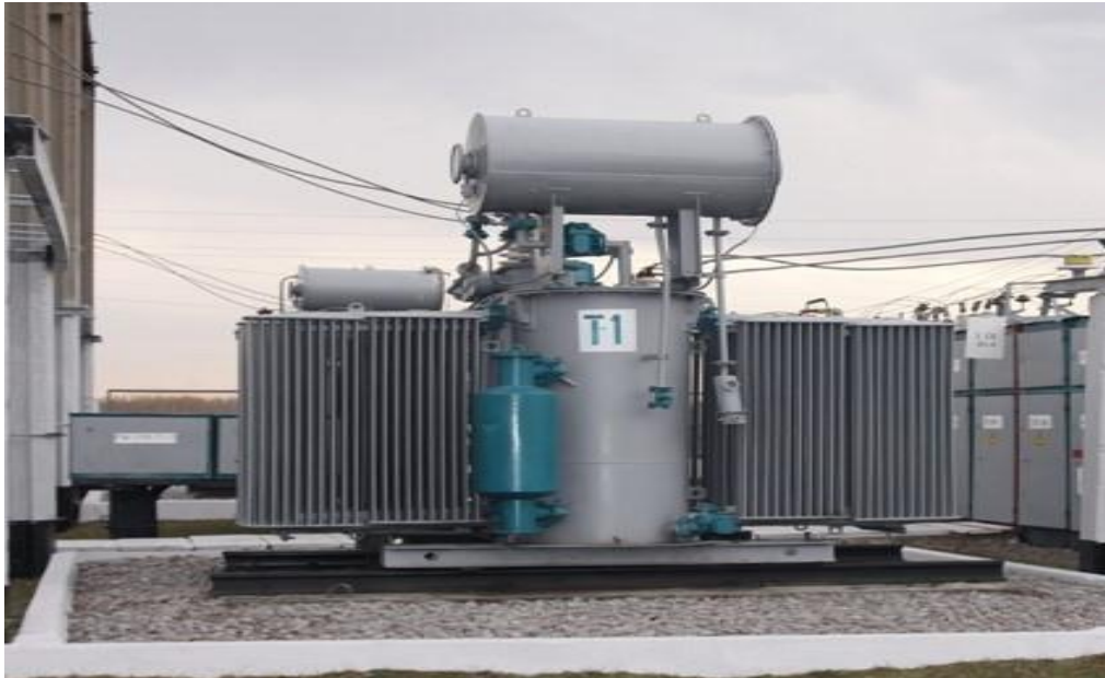
Figure 3.7 transformer used in power plant
