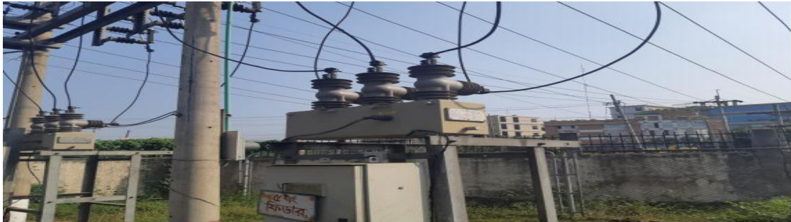
Figure 4.10: Feeding system of transformer in sub-station
