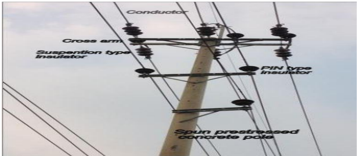
Figure 4.2: Fitting Of Distribution System
