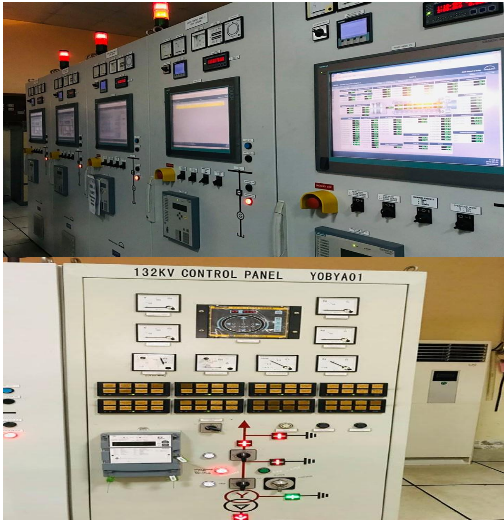
Figure 3.7.1: 132kv control panel
