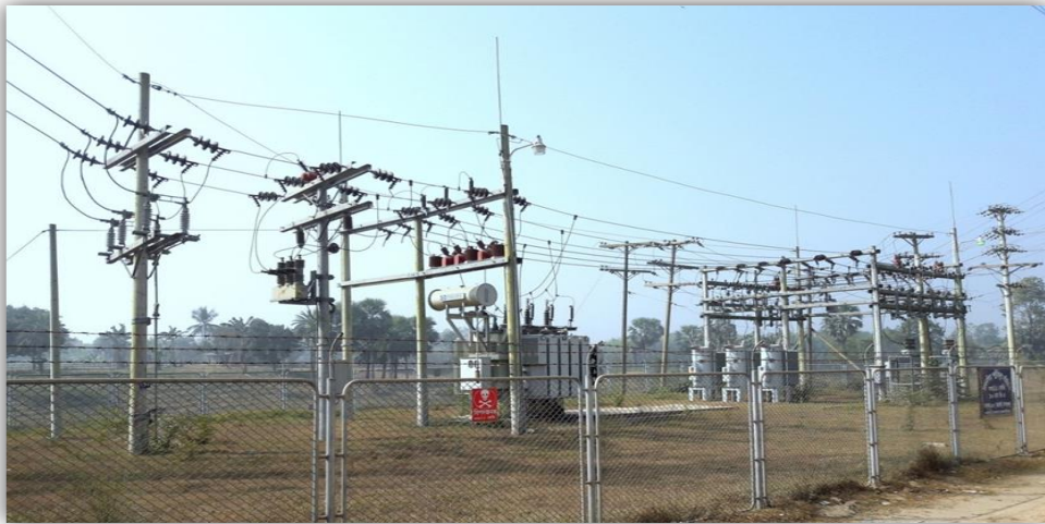
Fig 5.1: Sub-Station of BMCL
