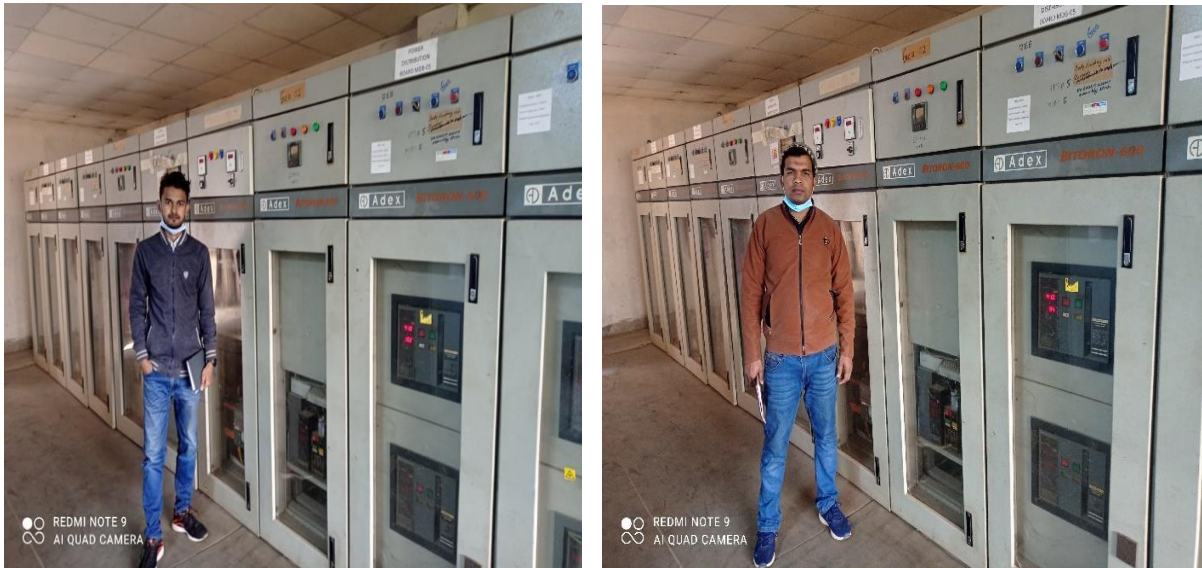
Fig 5.7: Power Distribution Panel Board
