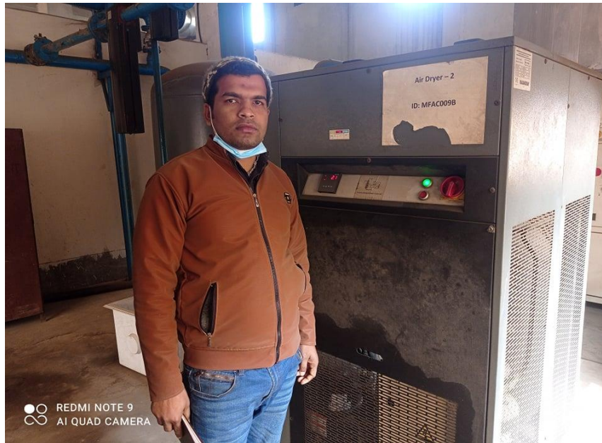
Fig 5.6: Air dryer 6.2 KW
