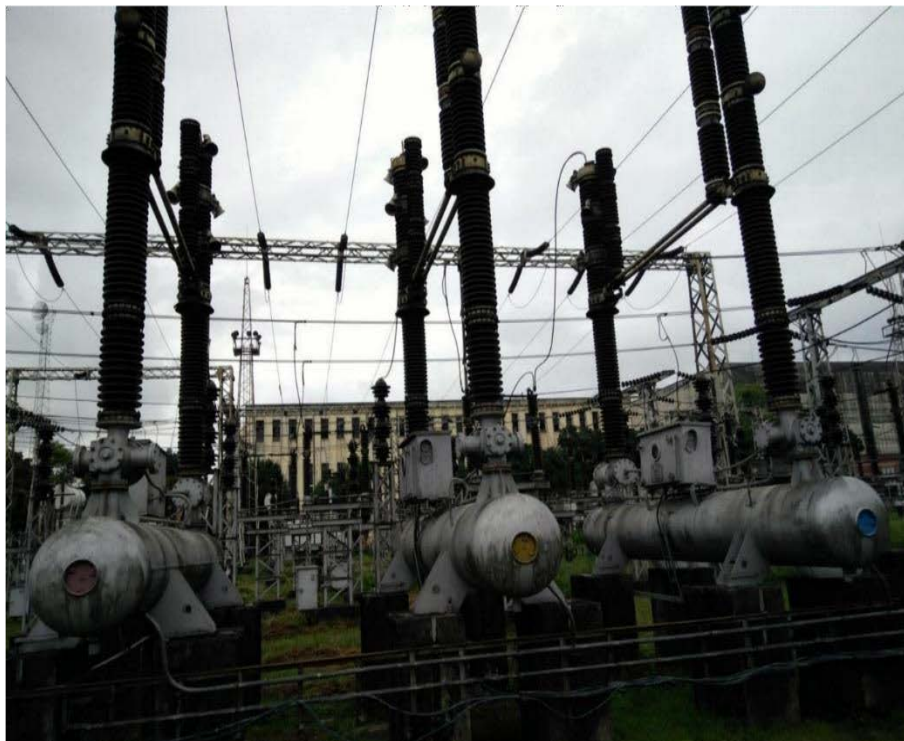
Fig. 6.6. SF 6 circuit breaker at GPS
