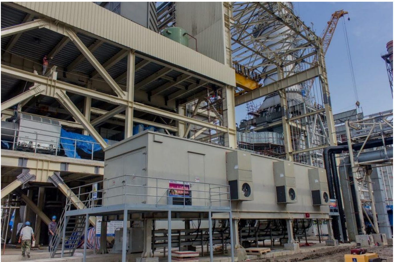
Figure 3.1: Gas Turbine Section
