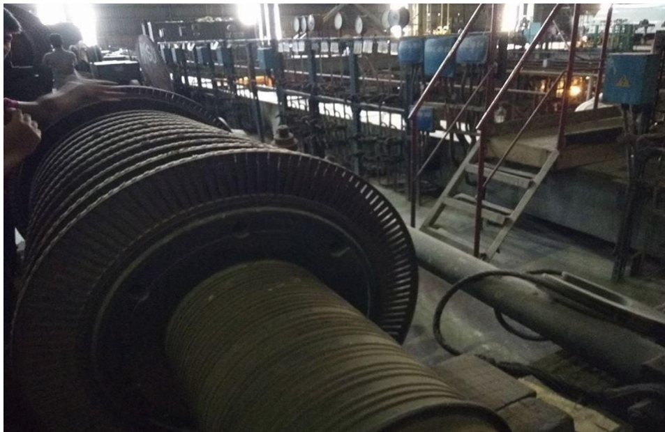
Fig. 4.2. Rotor of high pressure cylinder at GPS
