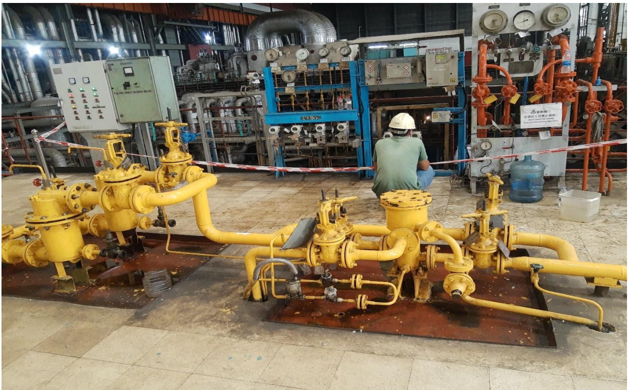
Fig: 5.6 Generator oil system
