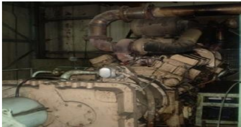
Figure.3.2 represents Diesel Engine to revolve the turbine
