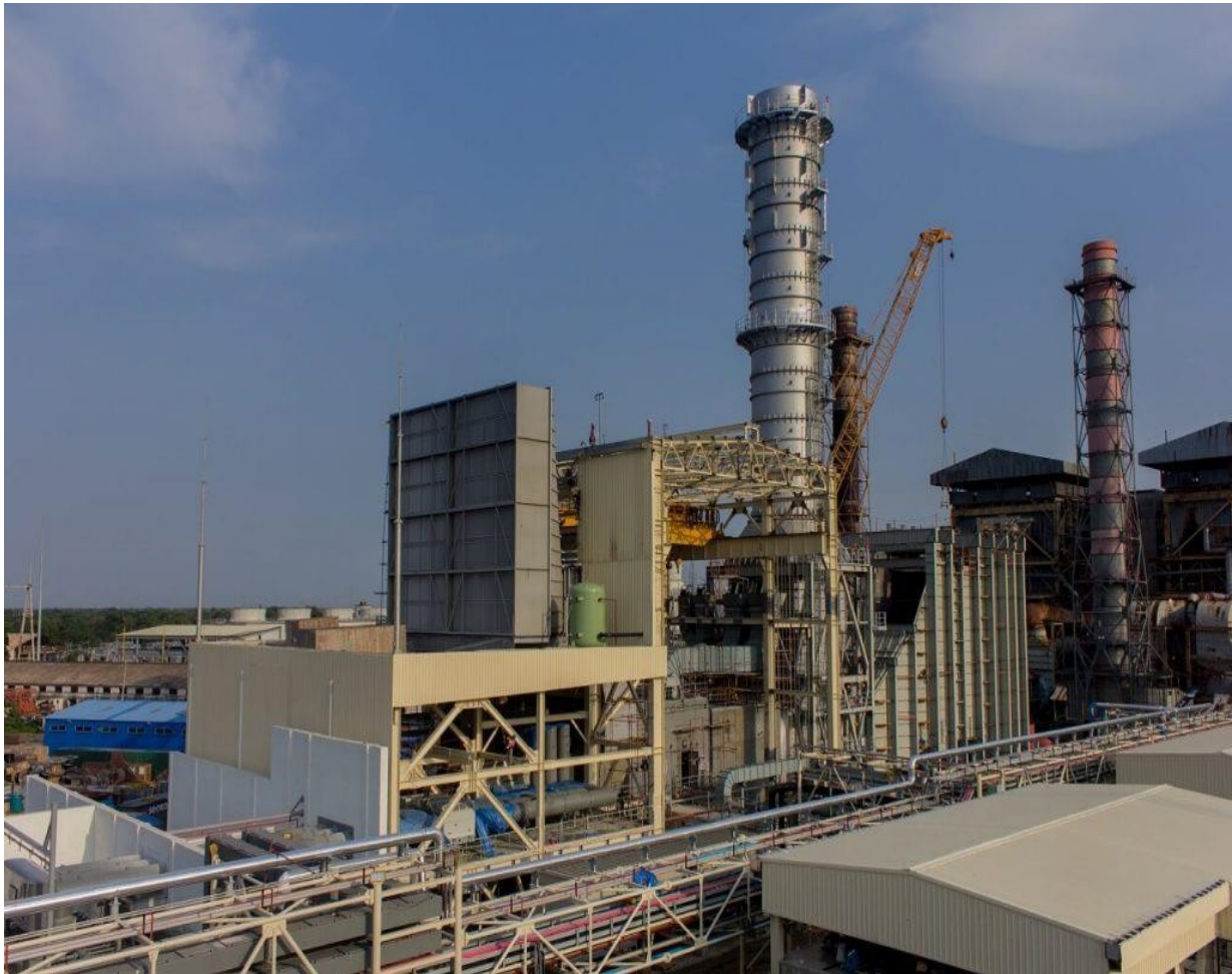
Fig. 2.1 Real view of 409 MW combined cycle power plant
