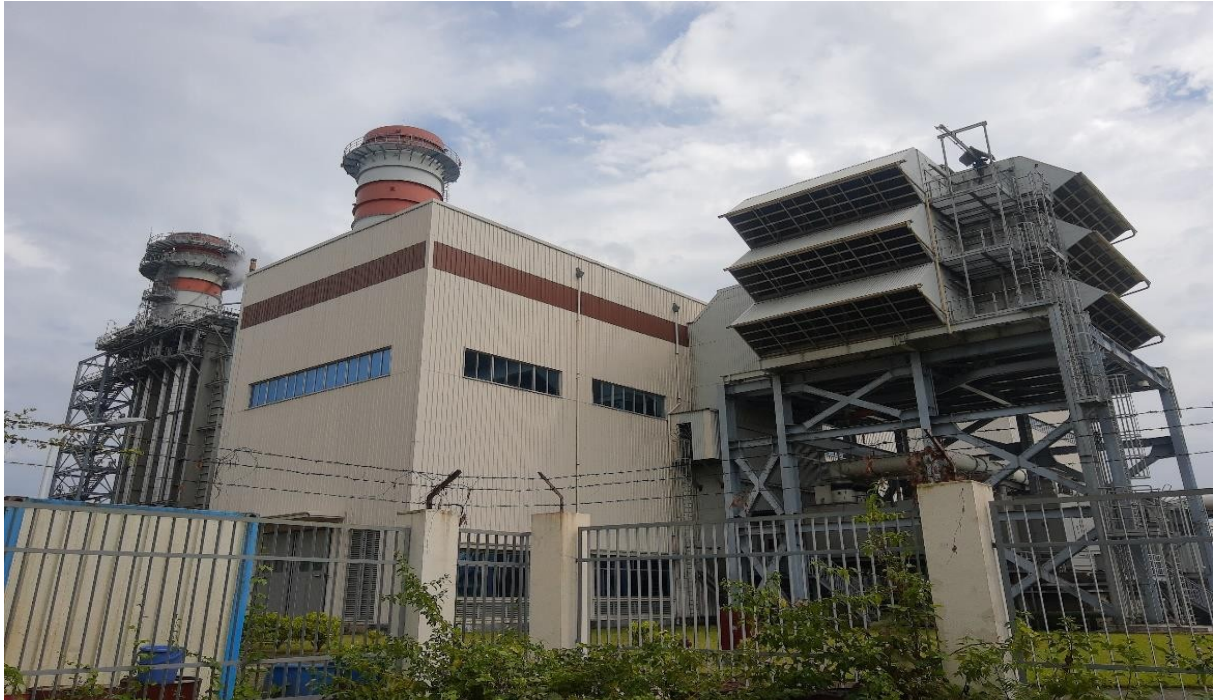
Fig. 2.3. Air inlet at GPS unit 4
