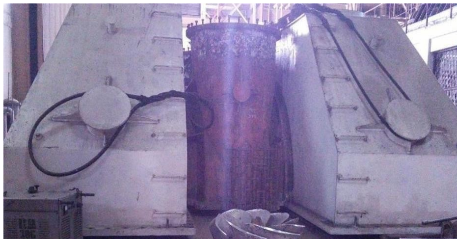
Fig. 4.5. Steam turbine condenser of unit-4 in GPS
