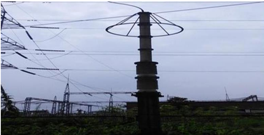
Fig. 67. Lightning arrester at GPS
