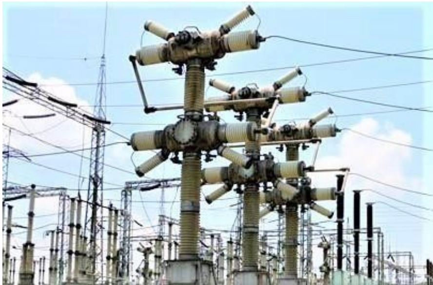
Fig. 6.5. Air blast circuit breaker at GPS
