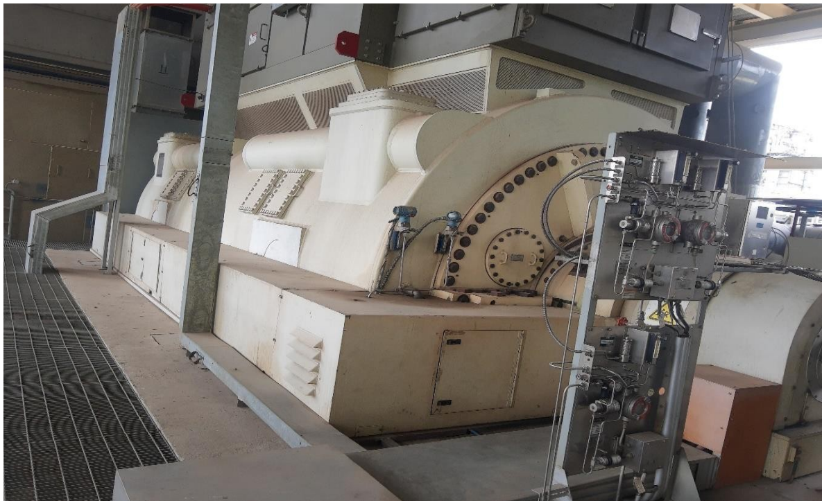
Fig. 5.2. Gas turbine Generator of unit-4 at GPS
