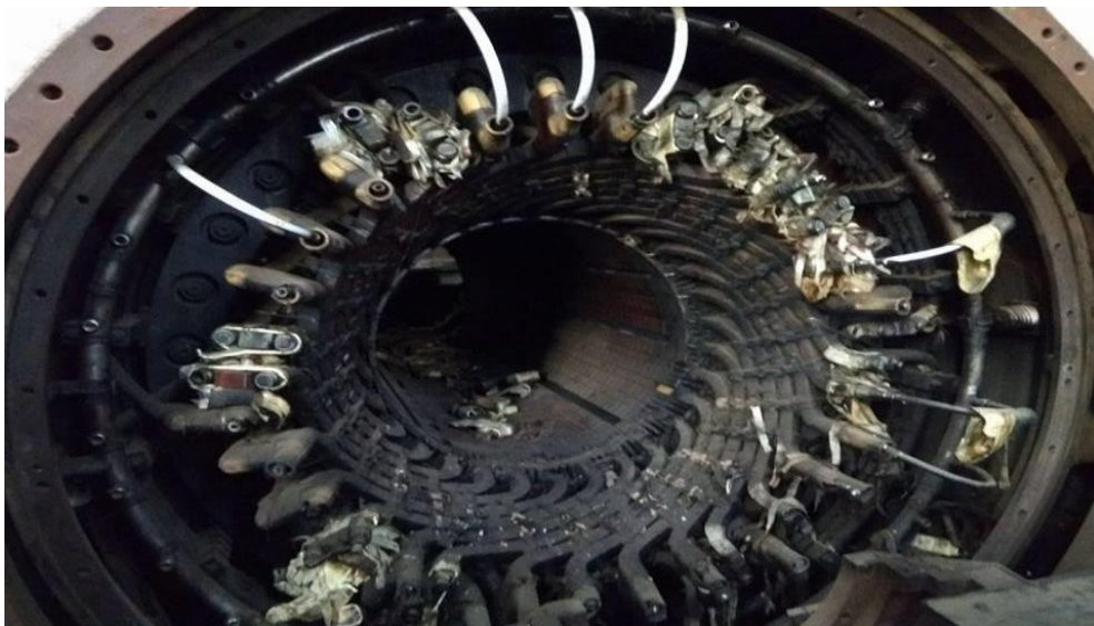
Fig. 5.3. Stator of generator at GPS
