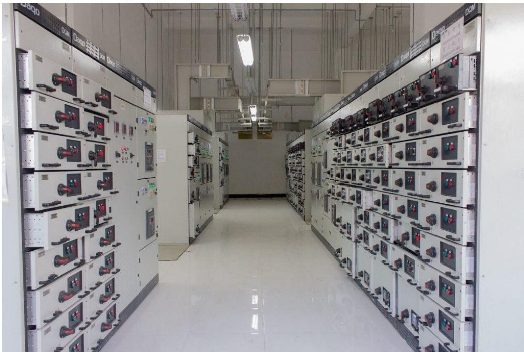
Fig. 7.1. Electric control room unit 4
