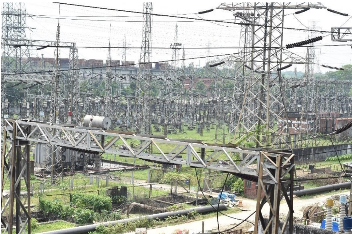
Fig. 6.1. Substation at GPS
