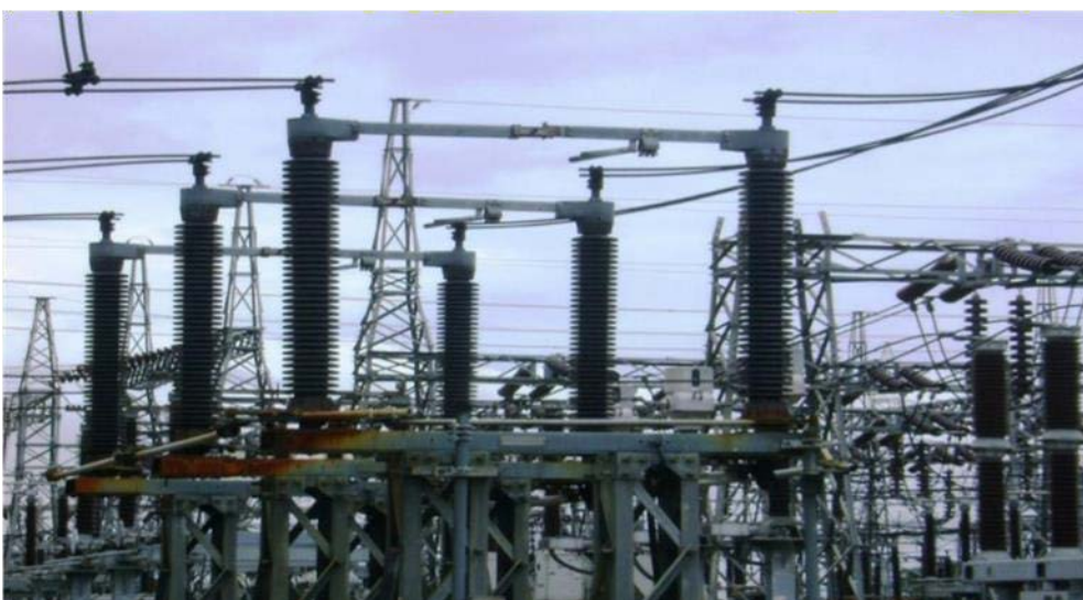
Fig. 6.9. Isolator at GPS
