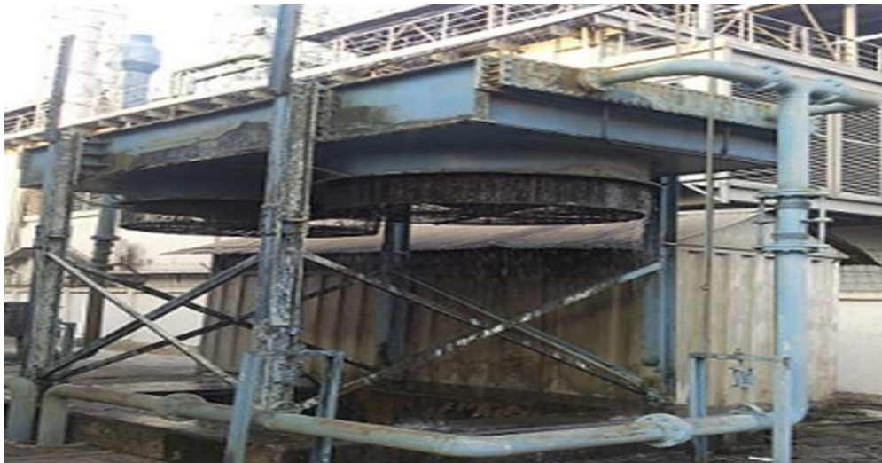
Figure 3.5: Lube Oil cooling plant
