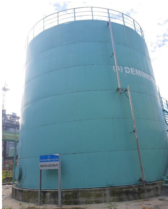
Fig no: 4.9 de-mineralized water tank
