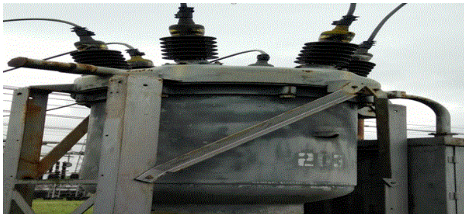
Figure6.4: Oil Circuit Breaker at GPS
