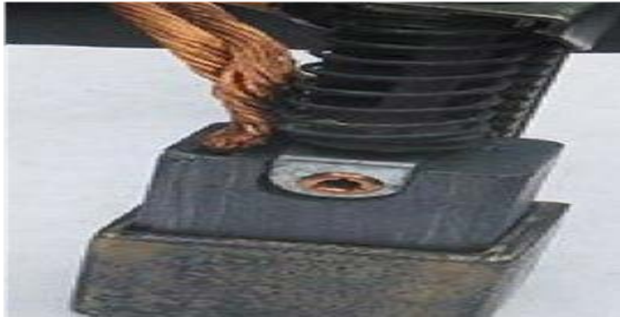
Fig. 5.5. Slip ring of generator at GPS
