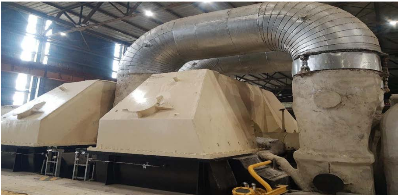
Fig. 4.1. Steam turbine section at GPS unit-4
