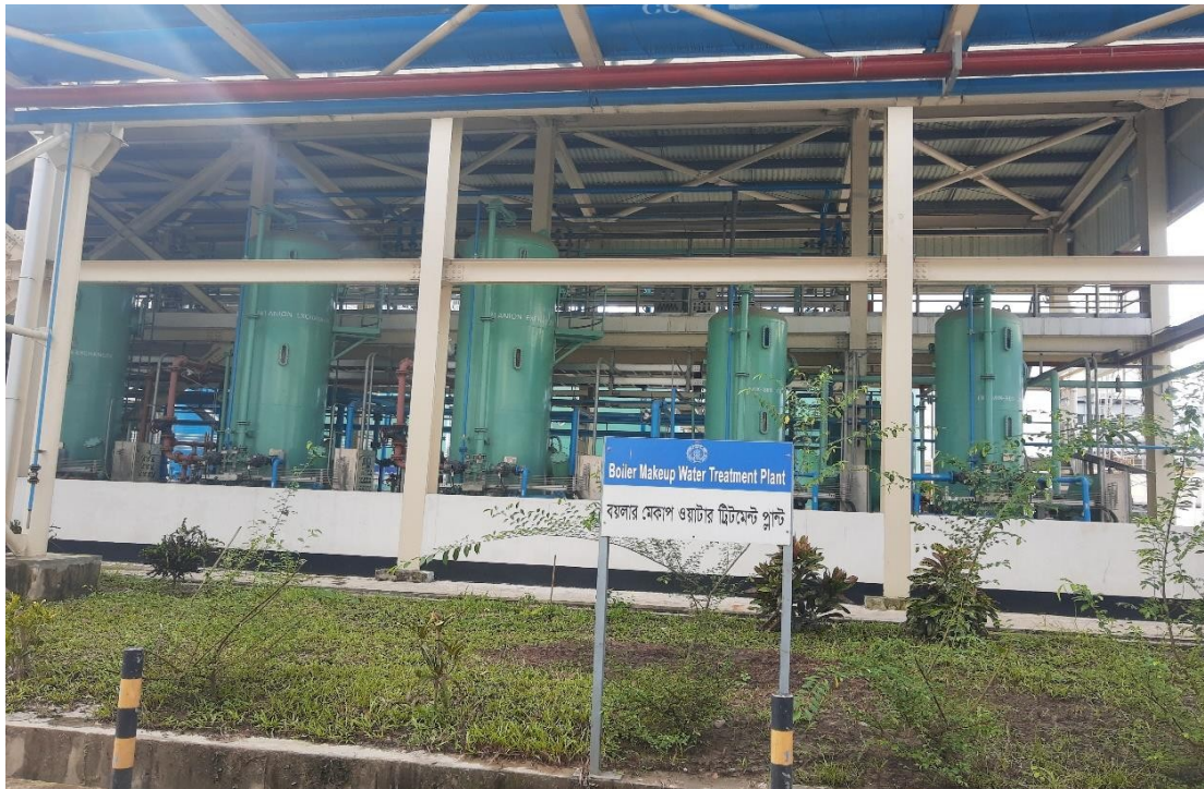
Fig. 4.7. Water treatment plant at GPS unit-4
