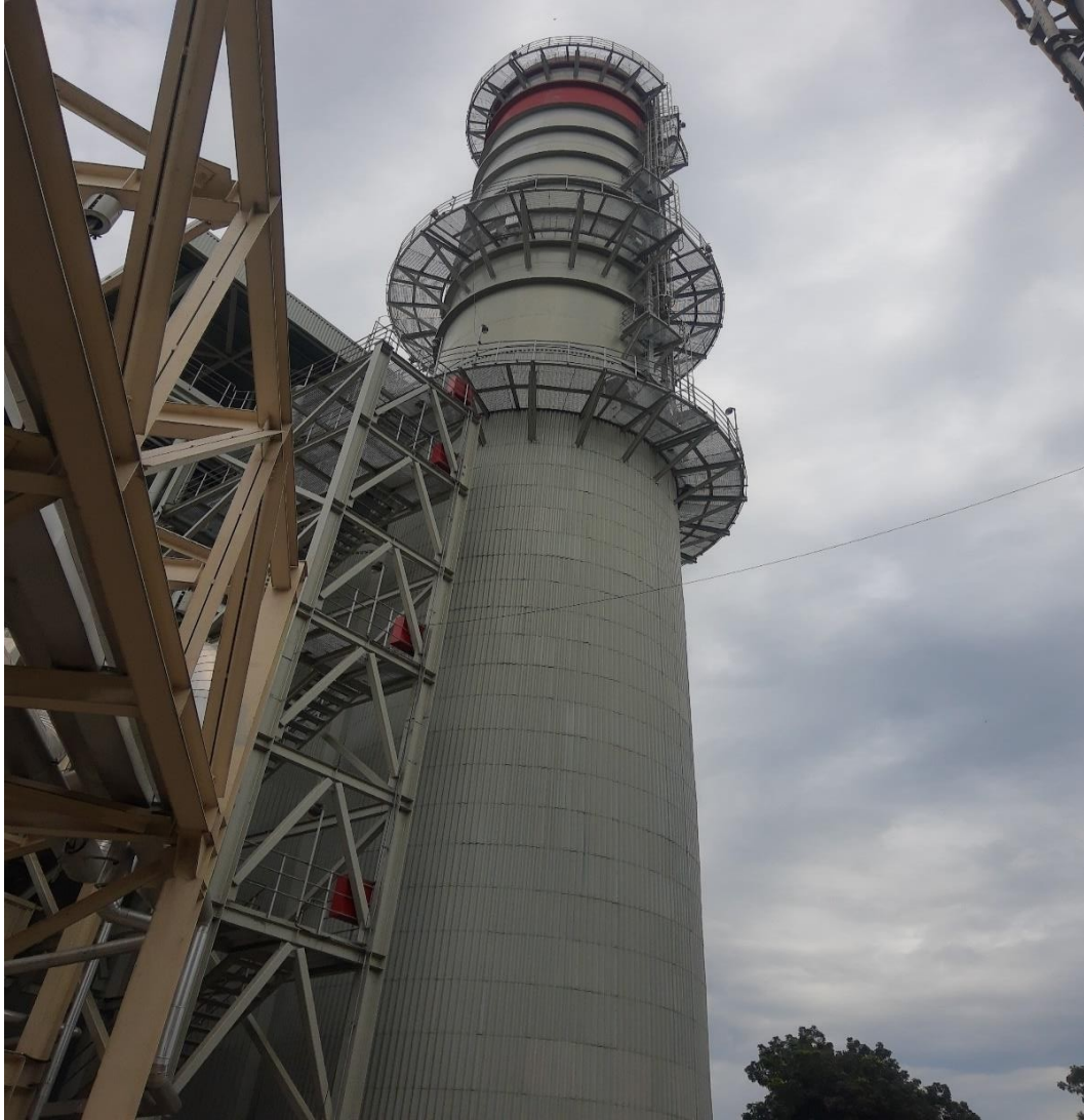
Figure3.3: Chimney of Waste heat recovery unit in combined cycle plant.
