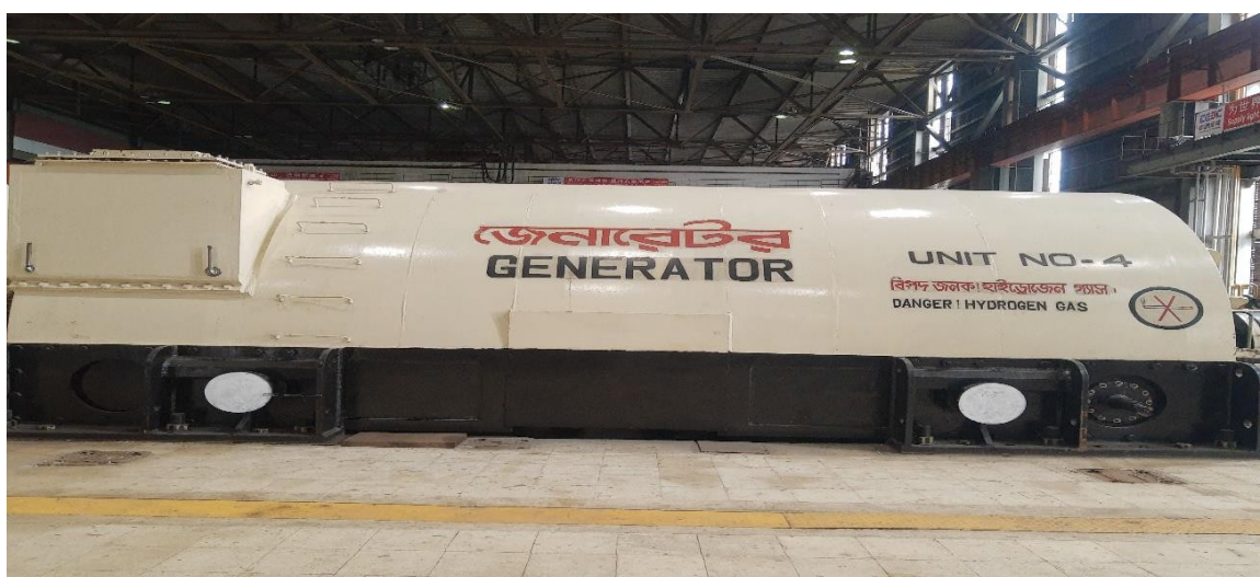
Fig. 5.1. Generator of unit-4 of GPS
