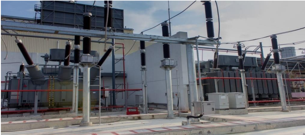
Fig.6.2. Bus bar at GPS
