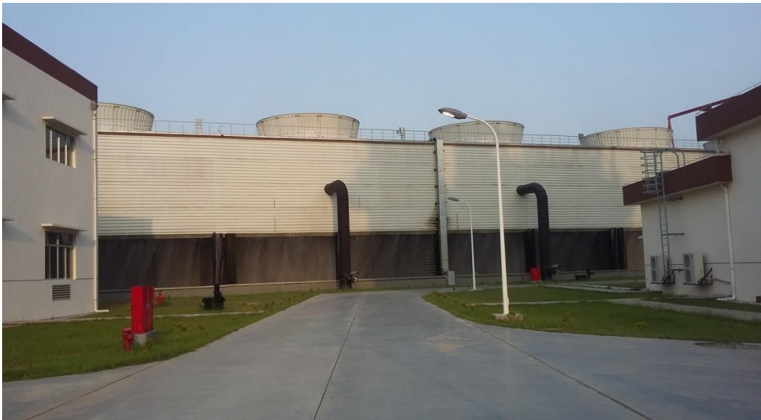
Fig. 2.5. Cooling tower at GPS Unit-4
