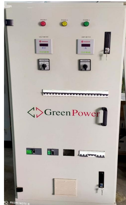
Fig 8.1: LT Switchgear Panel
