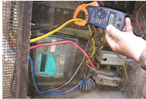
Picture2.2: Power theft test by manual [13]
