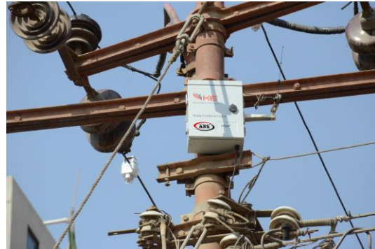
Photo 4.2: Data Concentrator Unit
