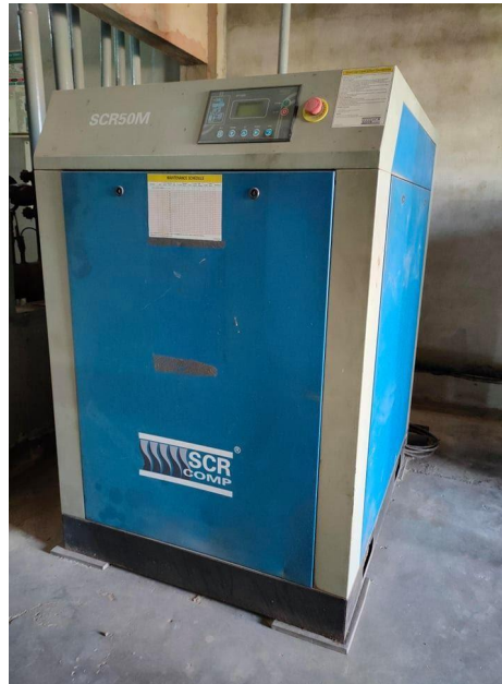
Fig: 3.1- SCR Compressors
