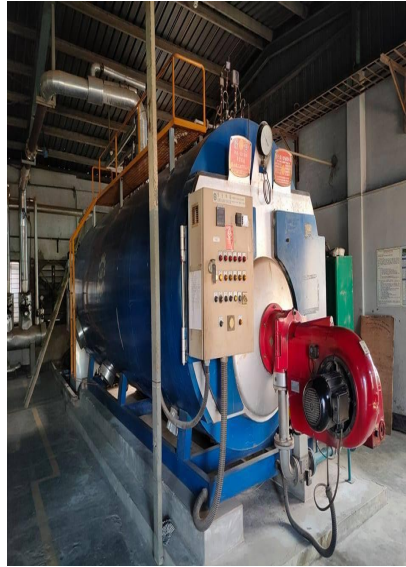
Fig: 3.2- Boiler Machine
